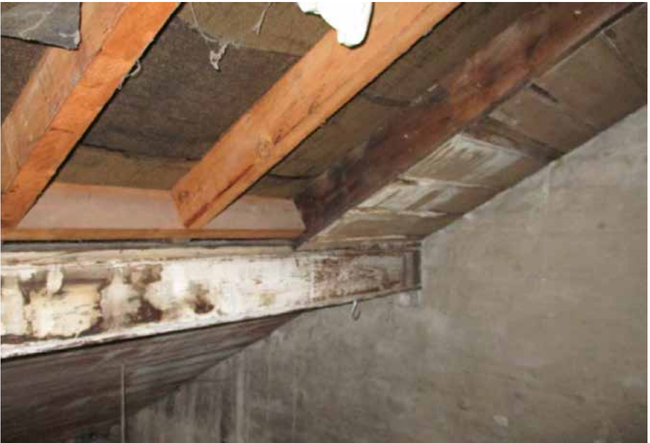
44. The appearance of the roofspace in room S3 in March 2019 (Client's own)
