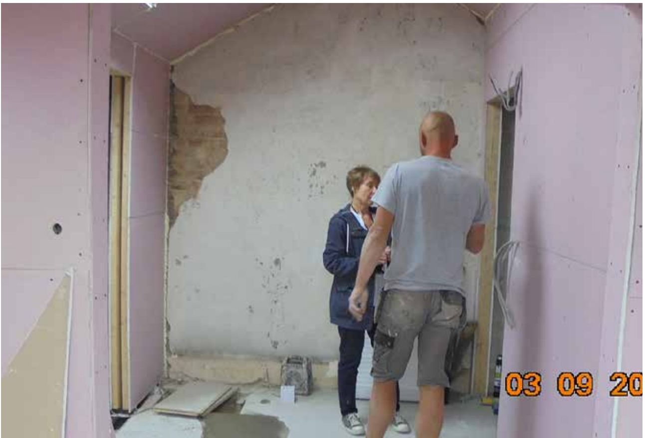
40. The unconsented doorways and platerboard added in room S1, September 2019 (Brighton and Hove Planning Archive)
