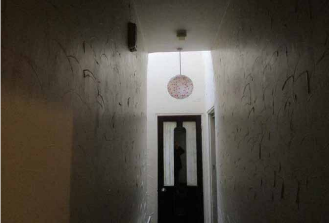
30. The altered four panel door to room F3 showing modern glazed toplights, March 2019 (Client's own)
