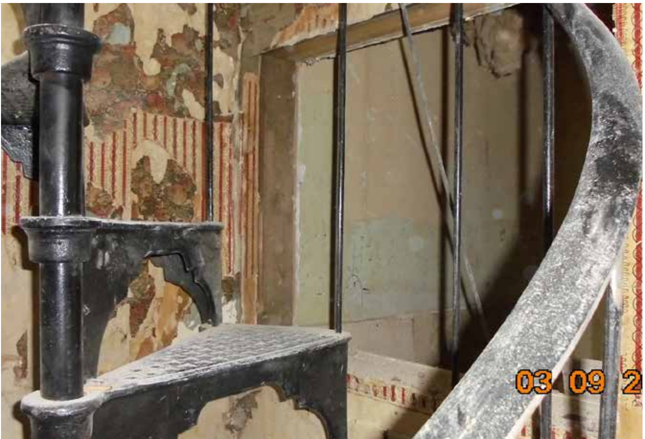
33. The original window opening to the north of F6, which was infilled as part of the unconsented works, September 2019 (Brighton and Hove Planning Archive)
