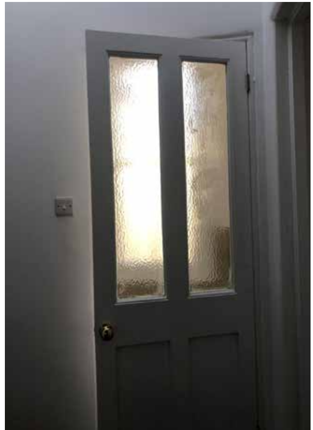
31. The unconsented altered glazed toplights in the door to room F3, February 2020 (Donald Insall Associates)
