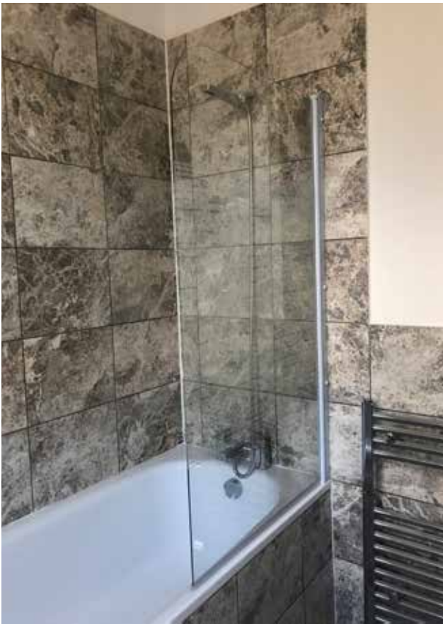
36. The unconsented partion wall and new bathroom fittings in room F4, February 2020 (Donald Insall Associates)
