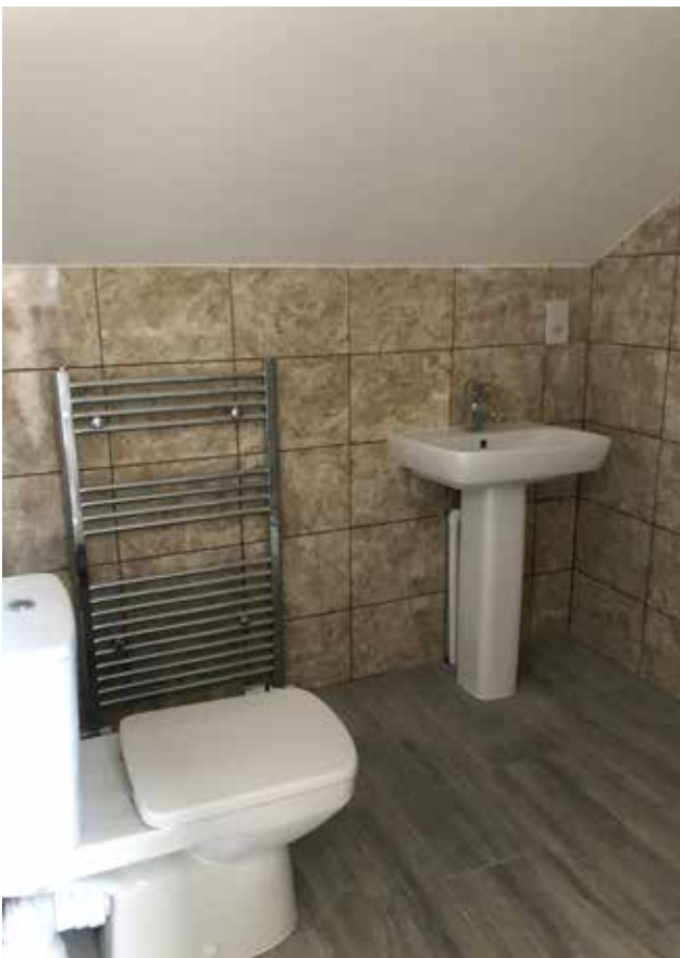
43. The unconsented bathroom fittings in room S2, February 2020 (Donald Insall Associates)
