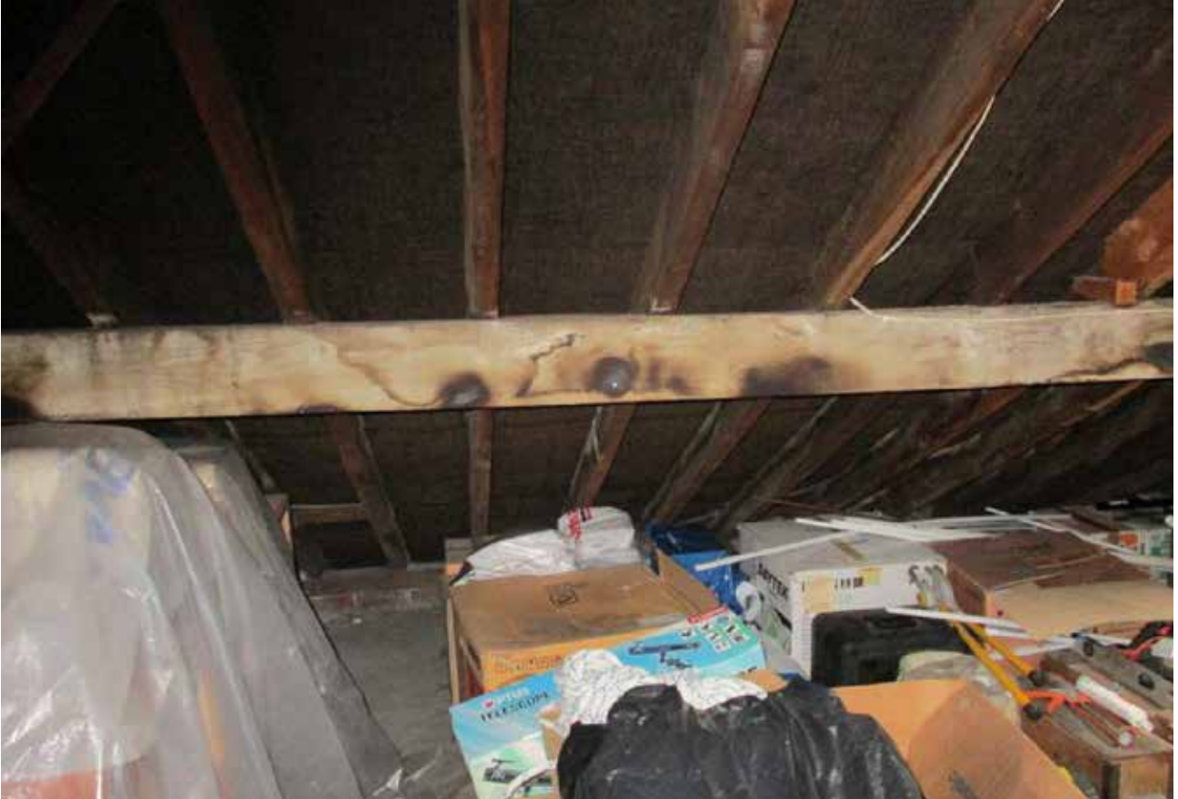
45. The appearance of the roofspace in room S3 in March 2019 (Client's own)
