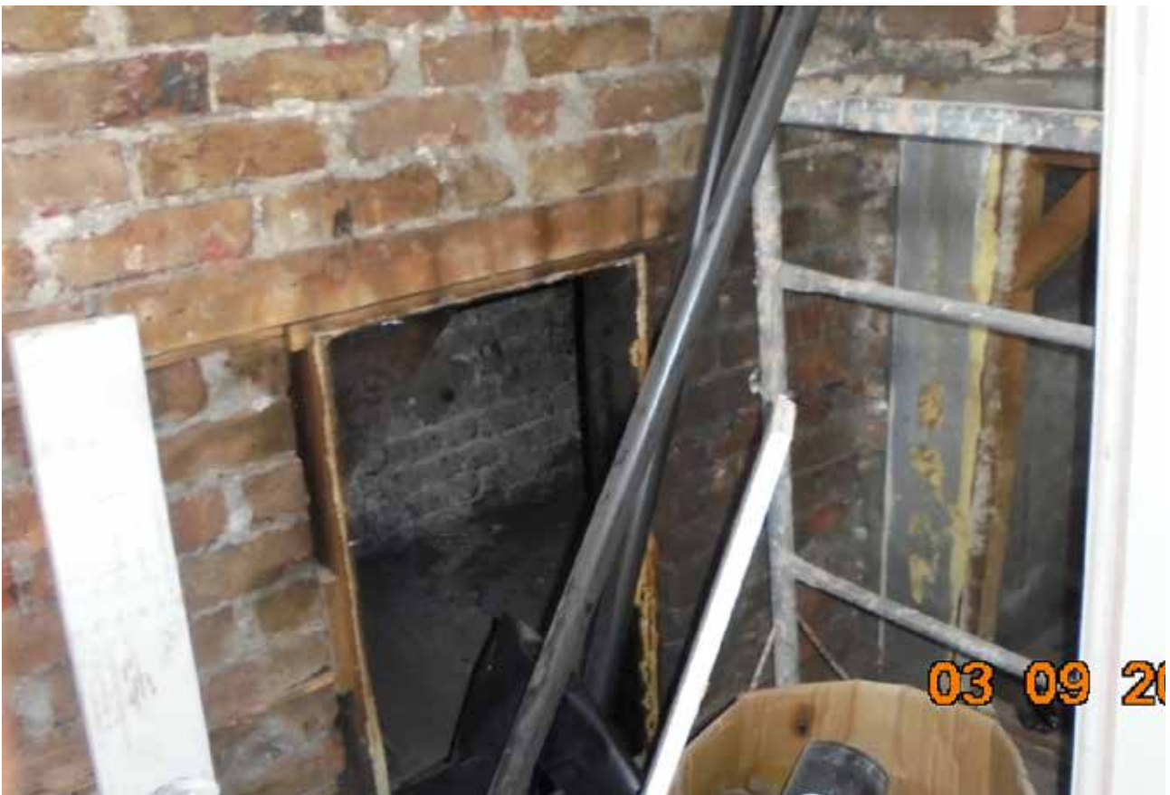
28. Brick interior of room G2 showing the temporary removal of the chimney piece, September 2019 (Brighton and Hove Planning Archive)
