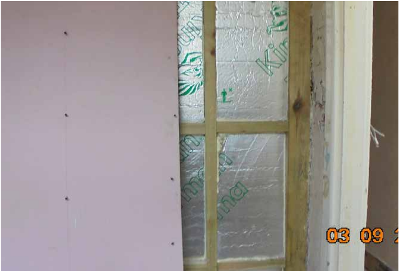
32. The unconsented partition constructed to subdivide room F4, September 2019 (Brighton and Hove Planning Archive)
