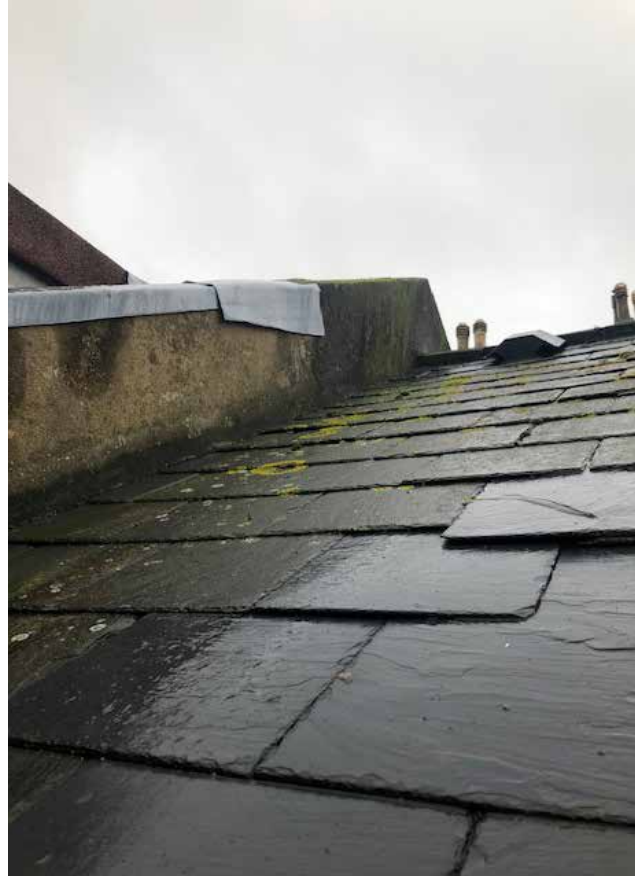
48. The unconsented extract fan on the north roof slope, February 2020 (Donald Insall Associates)
