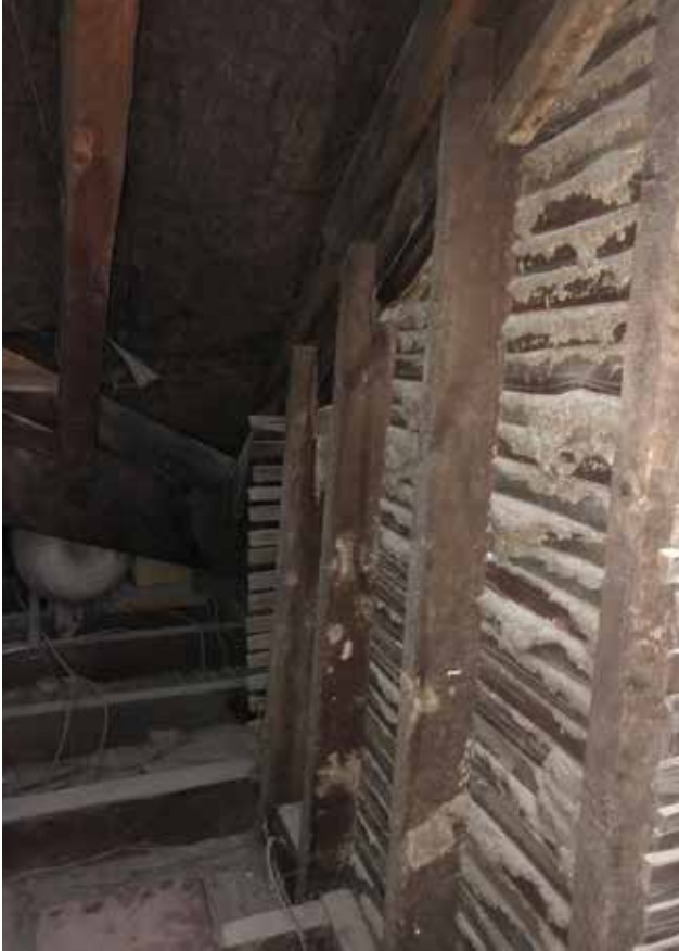
47. The retained roof structure under unconsented partitions in room S3, February 2020 (Donald Insall Associates)
