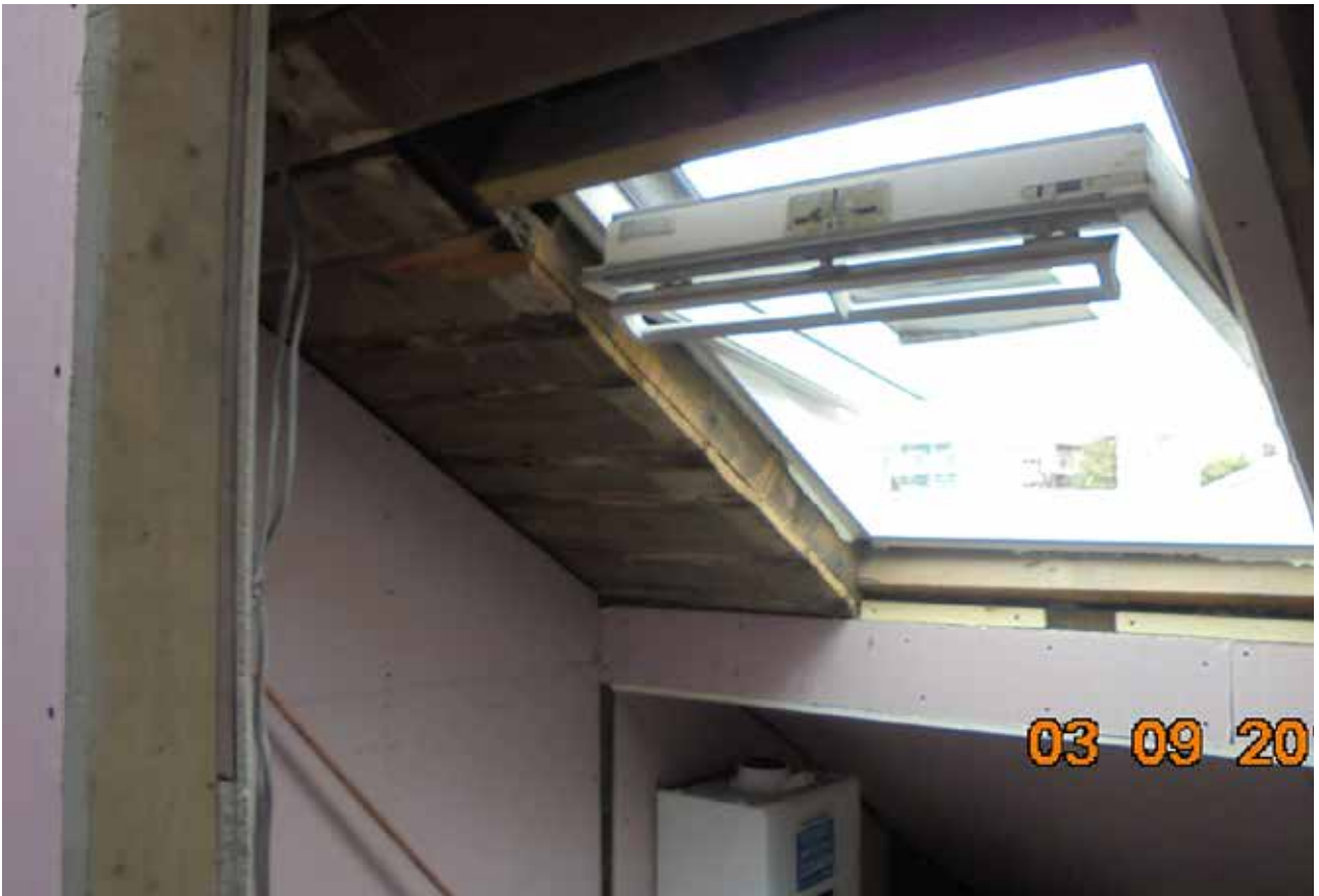
39. The unconsented rooflight added above the void in Room S1, February 2020 (Donald Insall Associates)
