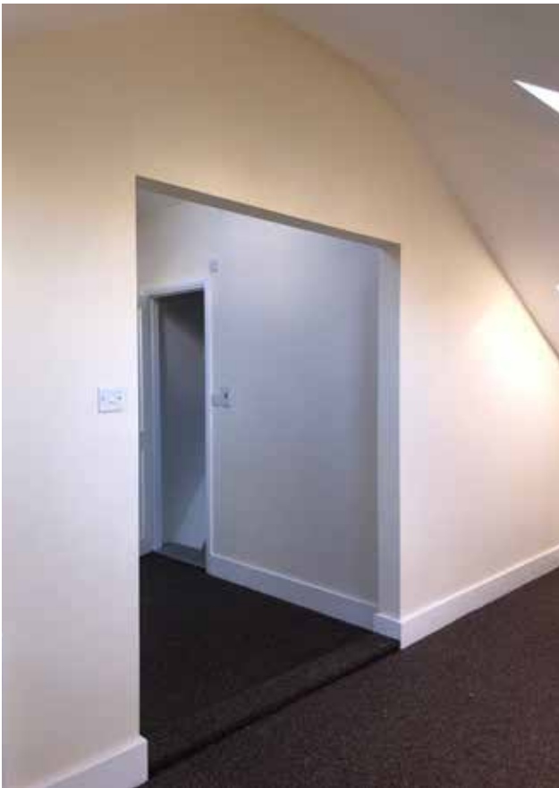
41. The unconsented double door opening to the west of room S1, February 2020 (Donald Insall Associates)
