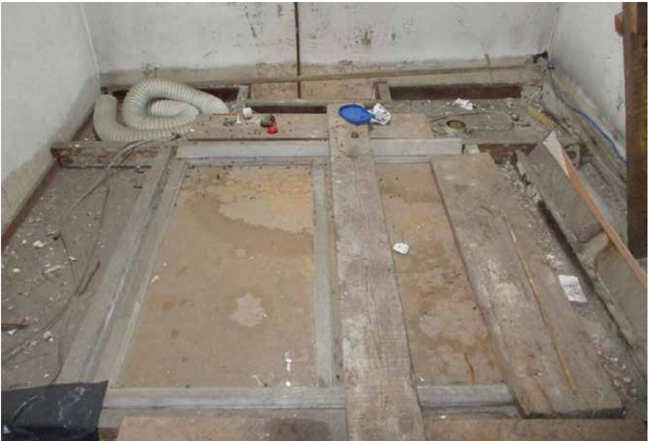
38. The late-20 th century floor over the former skylight in the ceiling of room F6, March 2019 (Client's own)
