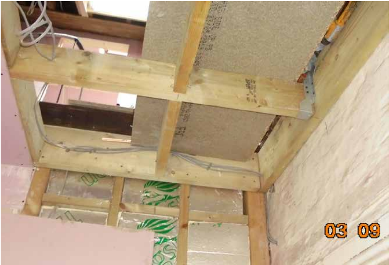
34. The unconsented infill of the former void above the late-20 th century spiral staircase in room F4, September 2019 (Brighton and Hove Planning Archive)
