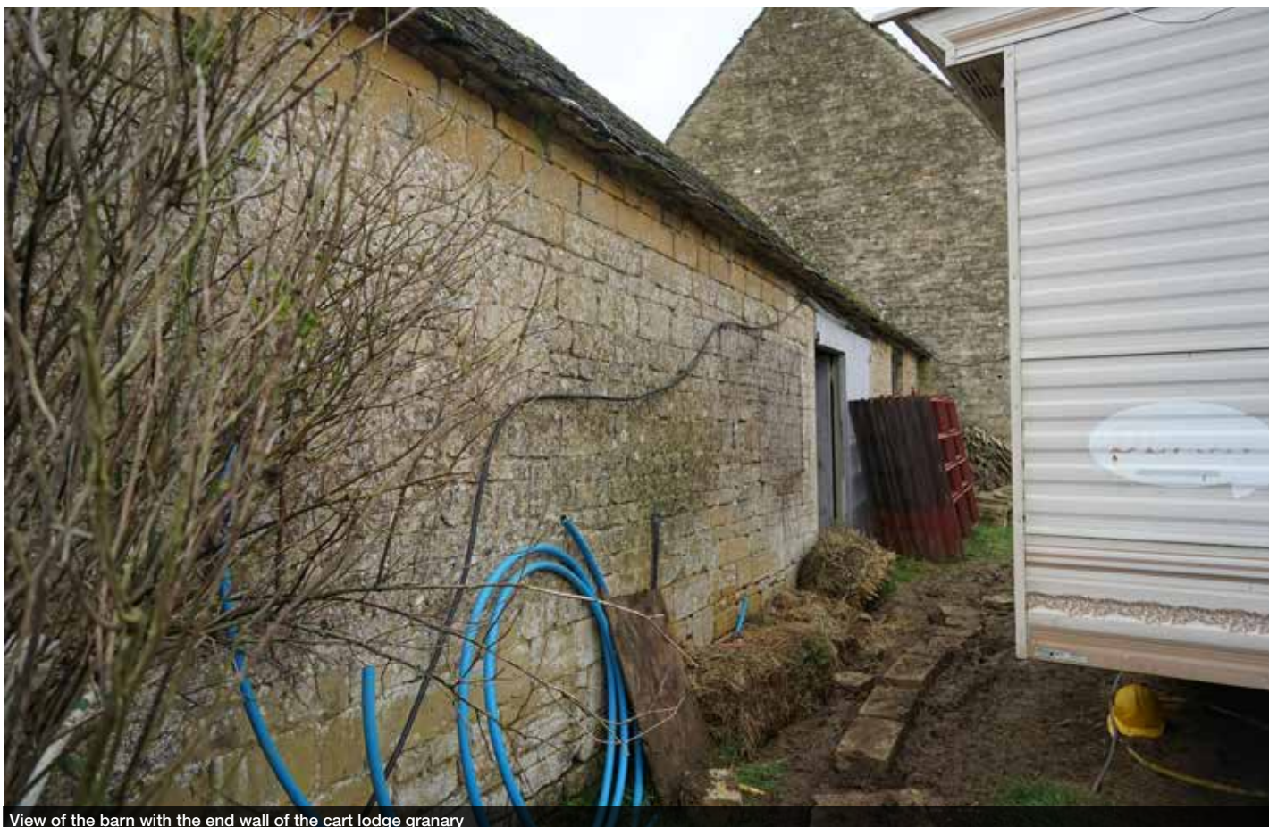
View of the barn with the end wall of the cart lodge granary
