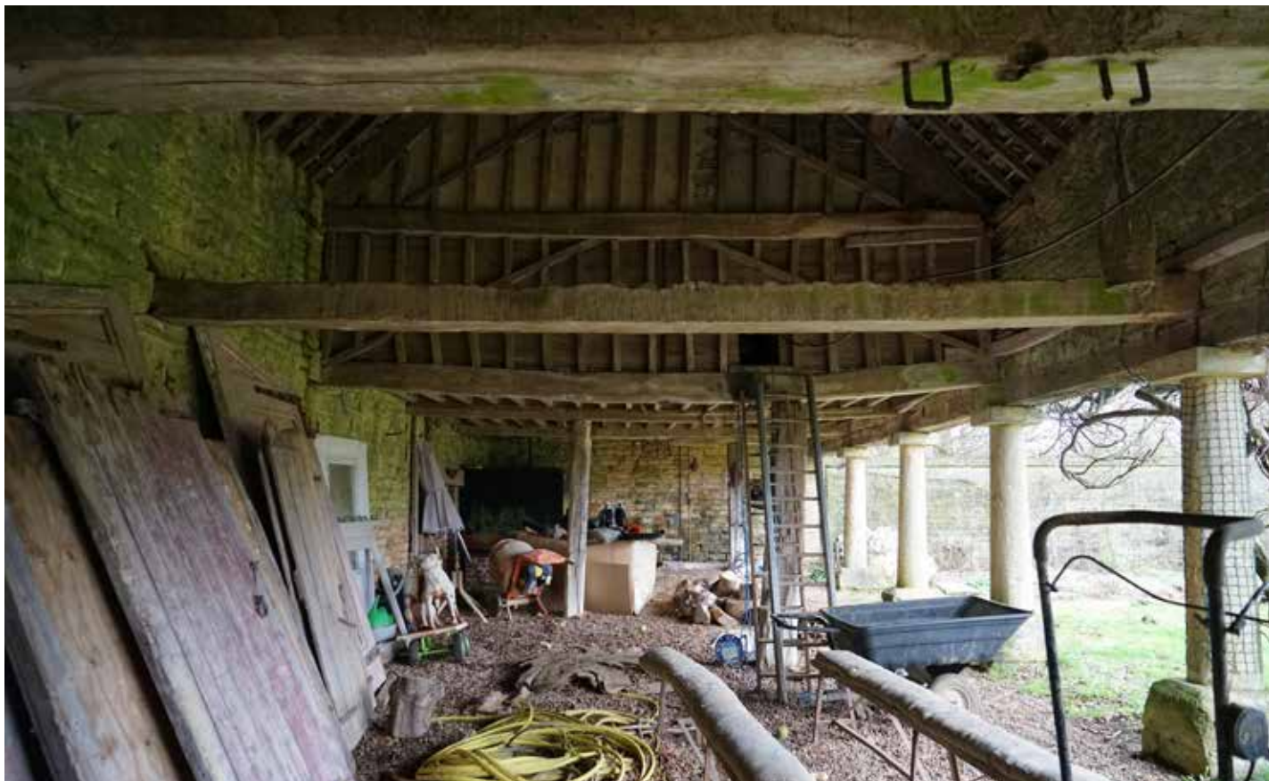
Interior looking north showing the stone bases, columns and pads, with beams spanning from above the columns to the rear wall. An infilled framed wall on the third bay encloses the first-floor granary
