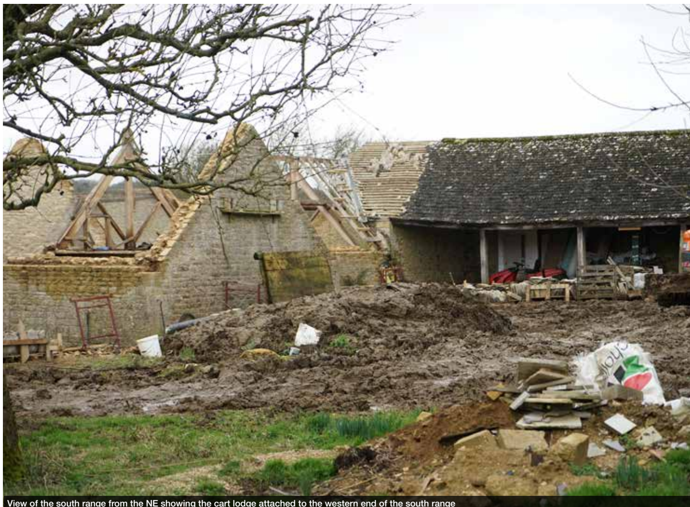
View of the south range from the NE showing the cart lodge attached to the western end of the south range
