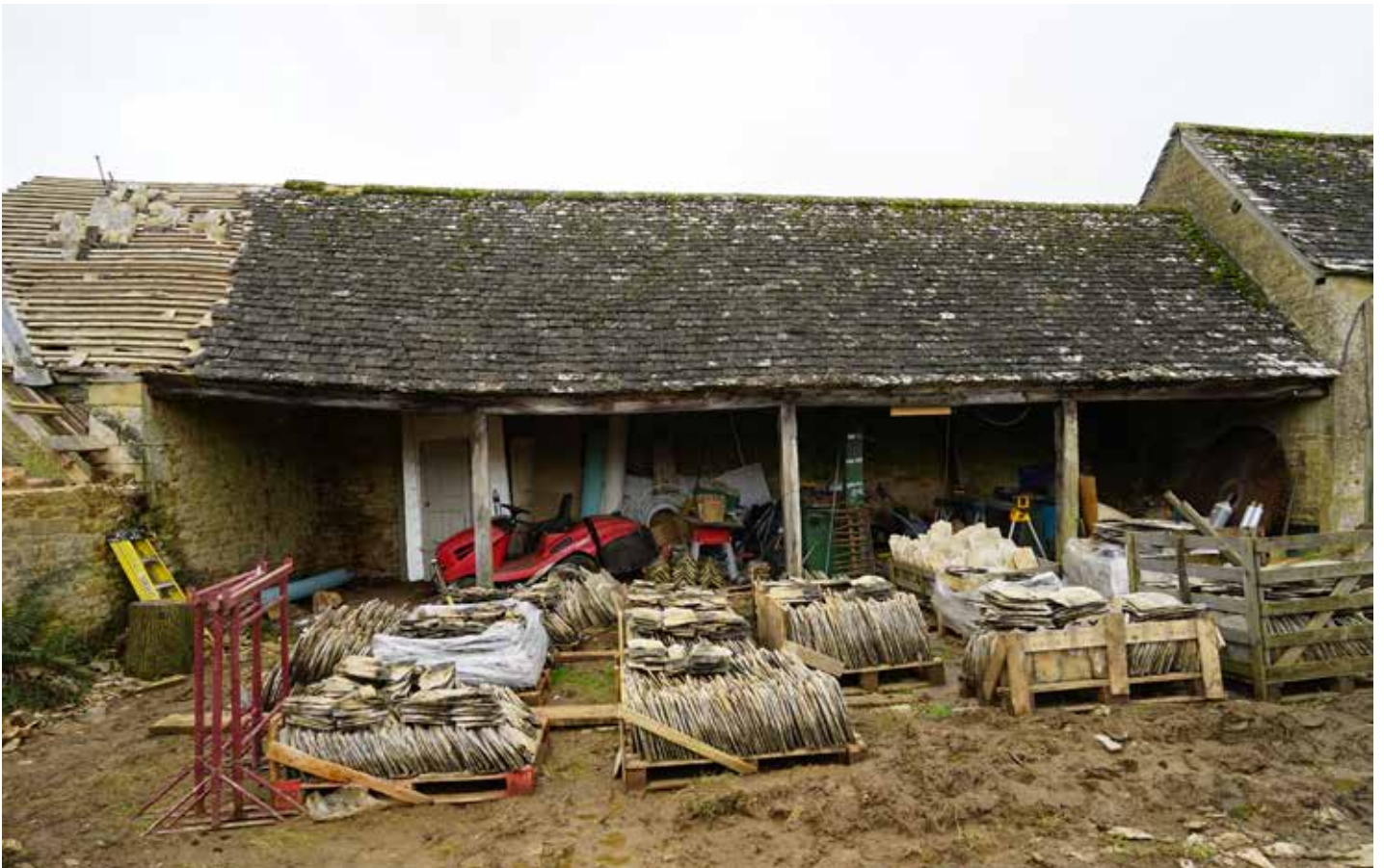
View of the second range of open cart lodges set below the roof line of the first showing re-tiling of the end bay
