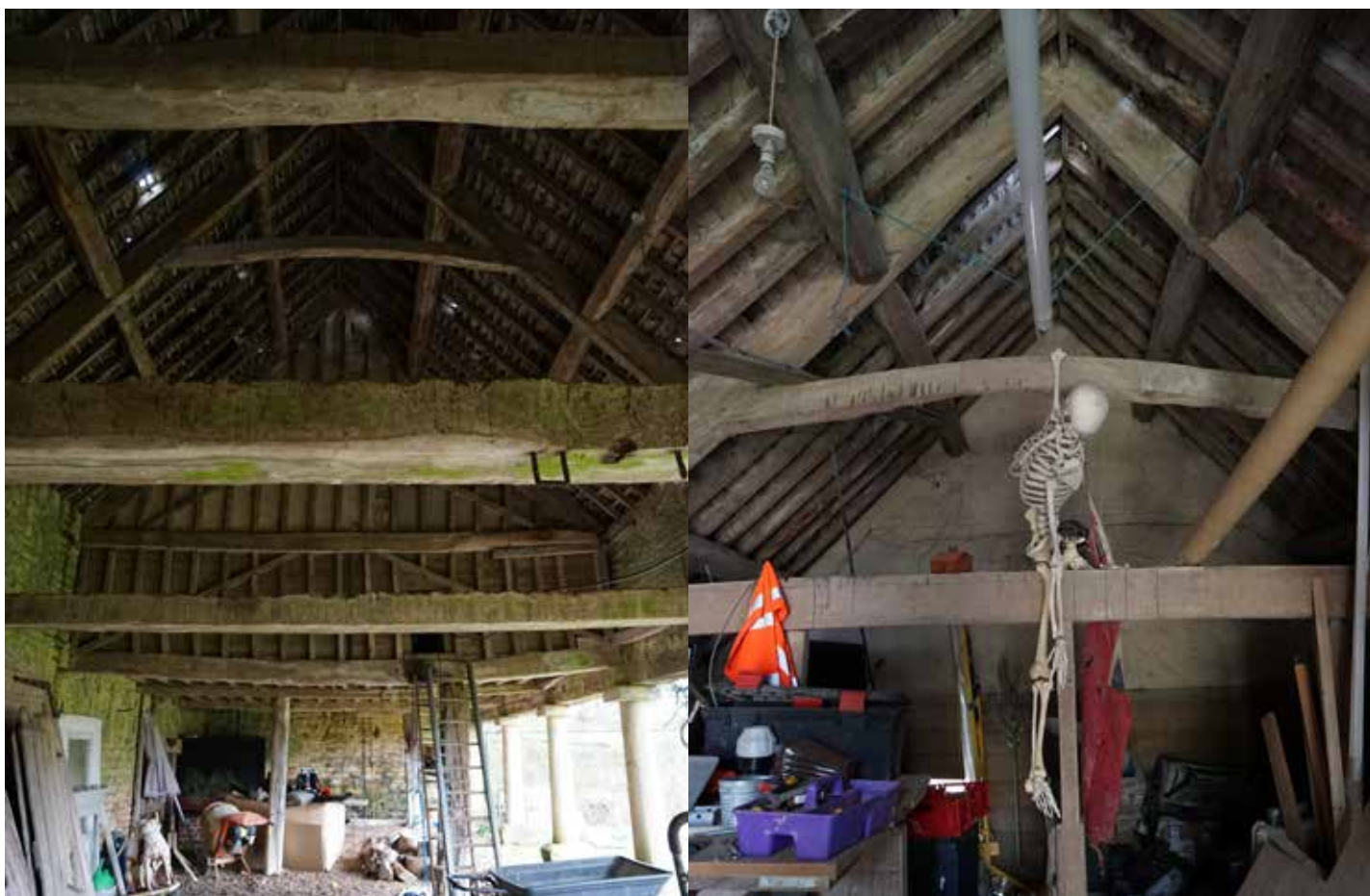
View of the roof framing looking north and inside the granary looking south. A double through side purlin roof with substantial principal rafters on each bay and a ridge board. A number of raised collars have later been inserted between the lower and upper purlins. On a number of the principal trusses
