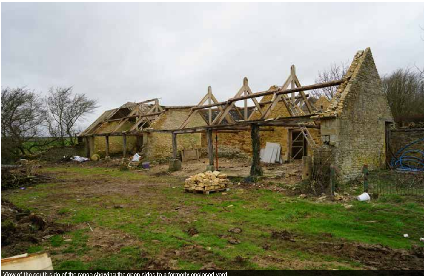
View of the south side of the range showing the open sides to a formerly enclosed yard
