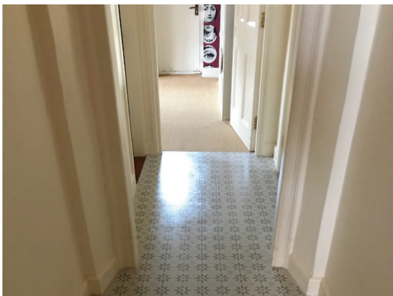
05: vinyl flooring & carpet to ground floor rooms and circulation spaces need to be lifted in order investigate the state of suspended floors. The ventilation grilles have been blocked in some areas and the installation of concrete floors in the South Eastern range will have prevented cross ventilation of the structure
