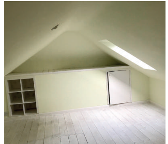
15b: first floor area of the annexe, this space will become part of the gym
