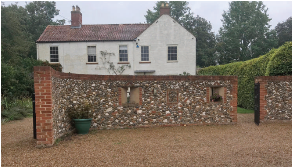
16: the modern garden wall between the house and the annexe to be removed to provide better vehicular access to the open cartshed
