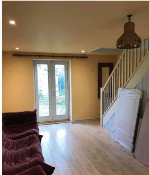
15a: Ground floor of the Annexe, the intention is to remove the ceiling/first floor to provide a vaulted open plan gym
