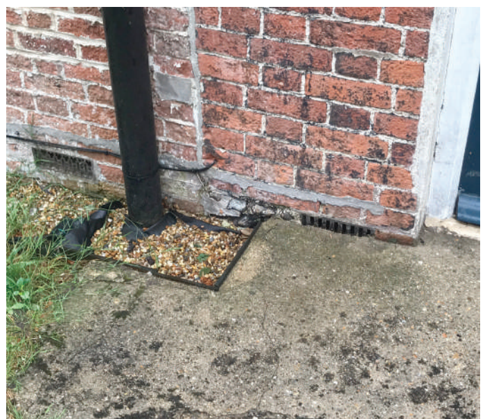
04: The ventilation grilles to the suspended floor have been blocked by internal
