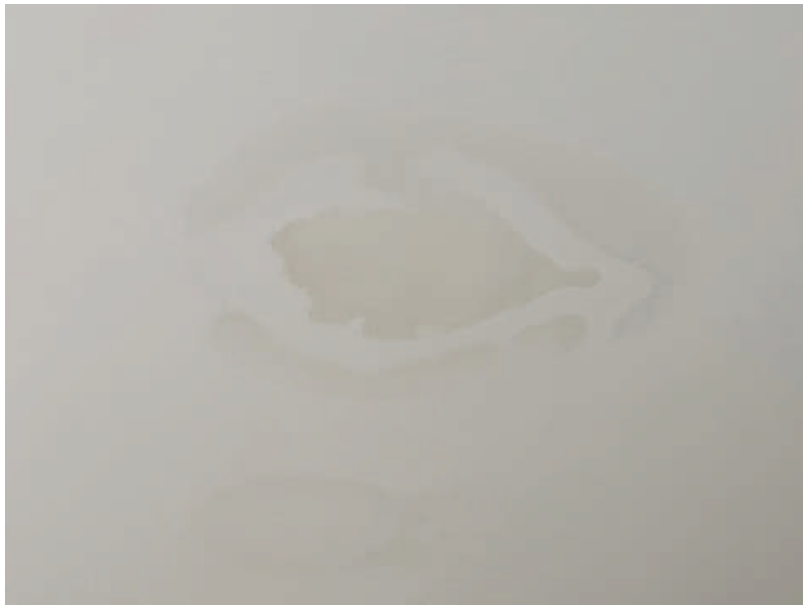
03: Stained ceiling of Master bedroom
