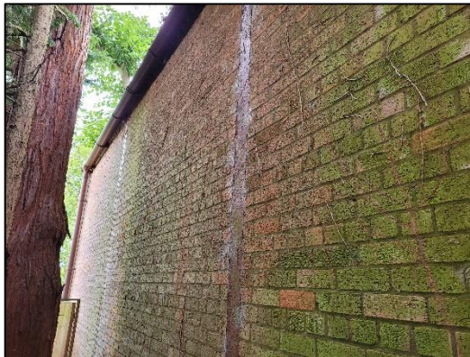
Plate 2: showing the brick wall that forms the rear (east) wall of the building.
