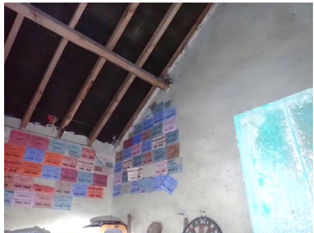
West end of Building A with small plastered room with bitumen felt sarking
