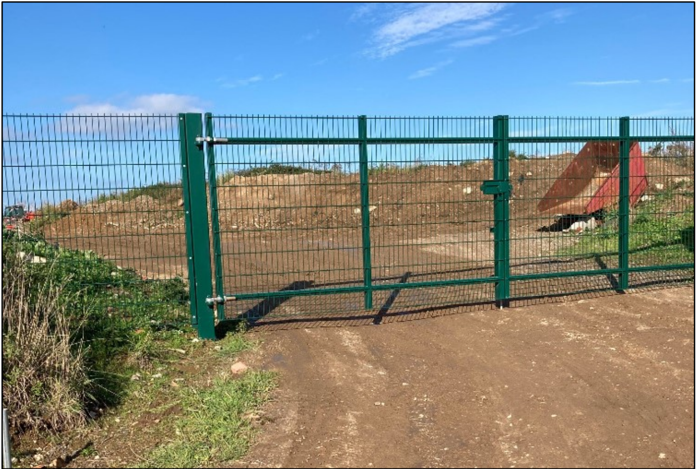
View into the site with the security gates and fence. The use of the site for the storage of materials and plant can be seen. The view also shows the height of the land behind the site.
