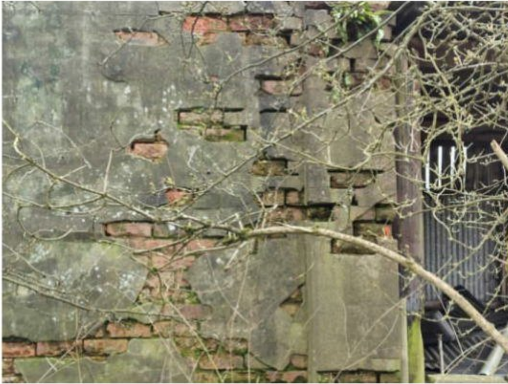
Figure 5. Damaged render obscured by scrub at northeast elevation.
