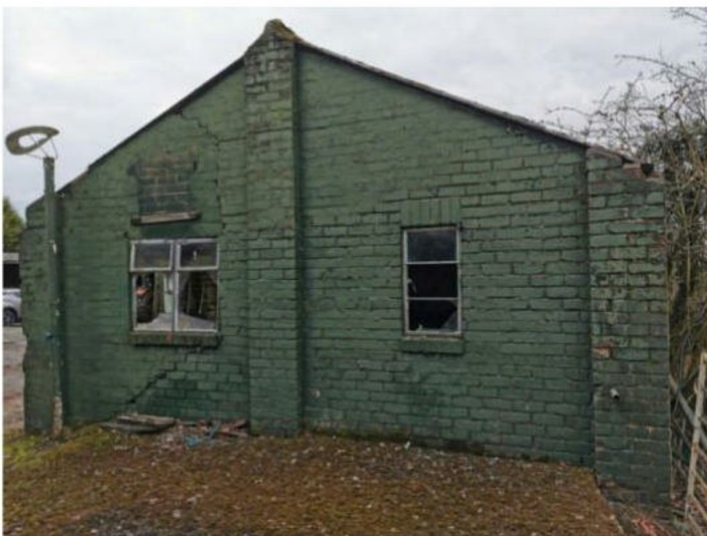
Figure 3. Southeast elevation showing crack in wall.
