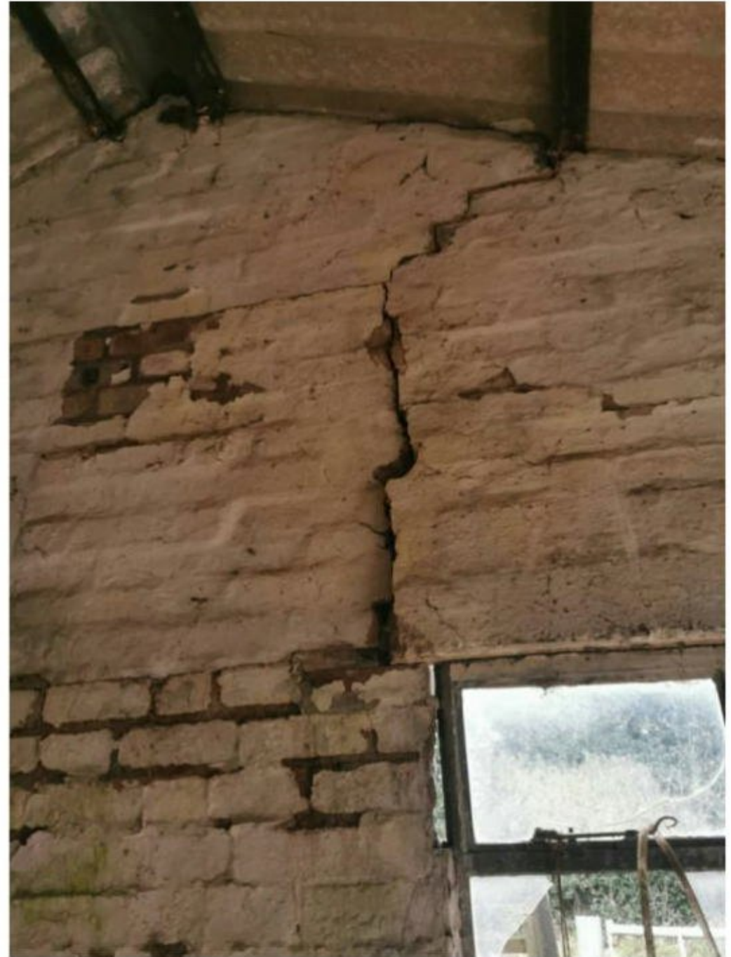
Figure 8. Crack in brickwork at southeast elevation
