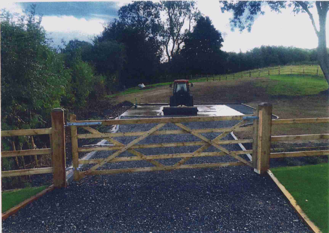
PHOTOGRAPH 3 - GENERAL VIEW OF THE EXISTING CONCRETE SLAB ON THE ADJOINING PLOT OF LAND.
