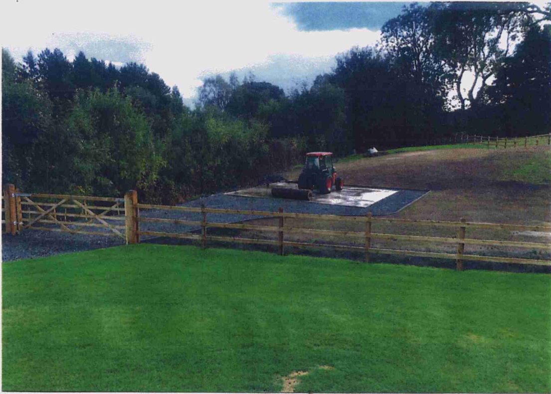
PHOTOGRAPH 4 - GENERAL VIEW OF THE EXISTING CONCRETE SLAB UPON WHICH IT IS PROPOSED TO CONSTRUCT A NEW STORAGE BARN.
