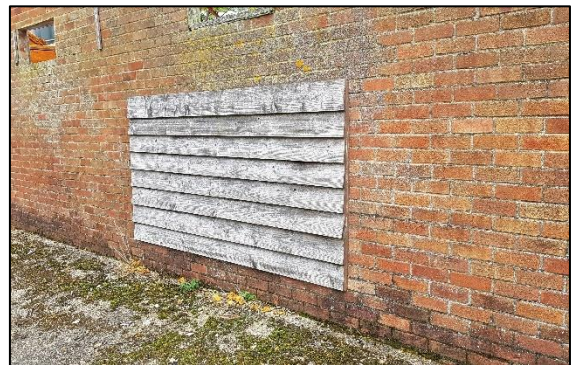
Figure 4: Small area of weatherboarding.
