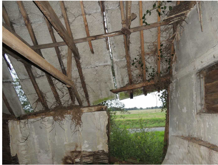
Photo 5: Note gap in NE wall
