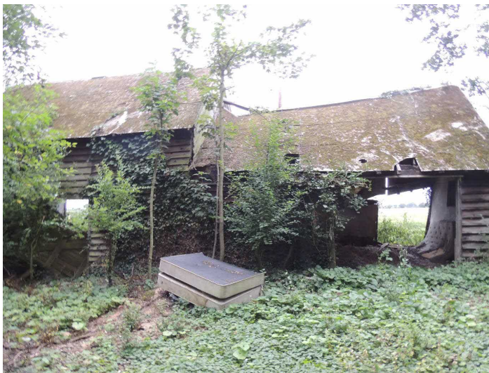
Photo 3: South-western elevation. Note gaps in walls
