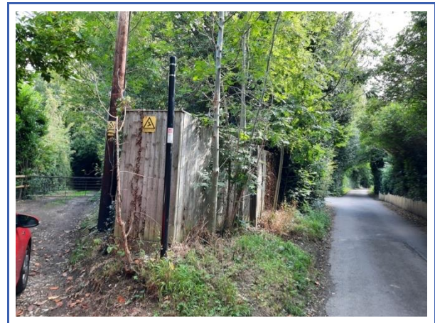
View of the electrical sub-station to the east
