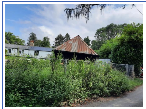
View of the barn on site with 1 & 2 Hartley Wood Corner Cottages to the north
