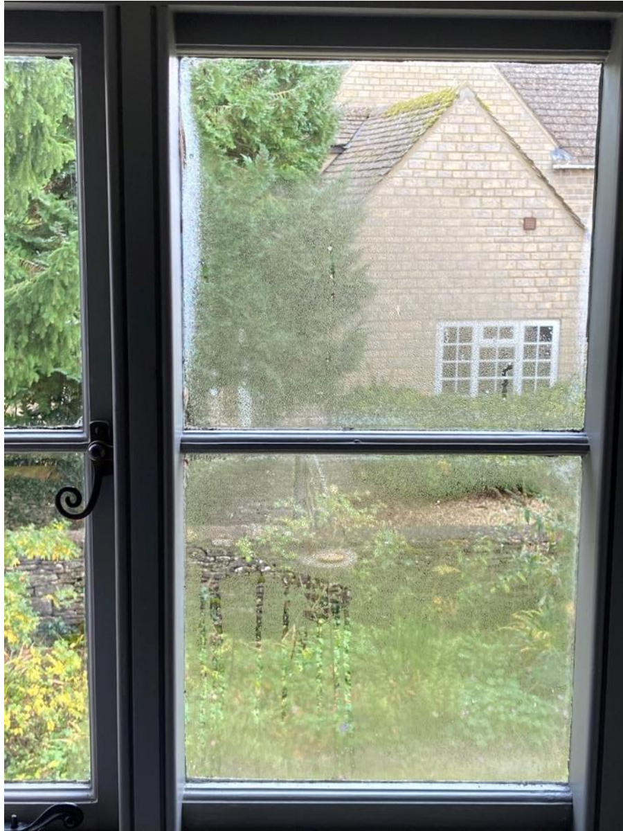
Interior bedroom showing typical condensation
