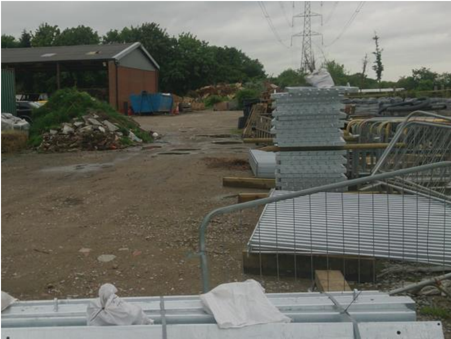
Material stored on site where the proposed car parking is proposed. View looking towards former barn to be demolished to make way for residential units
