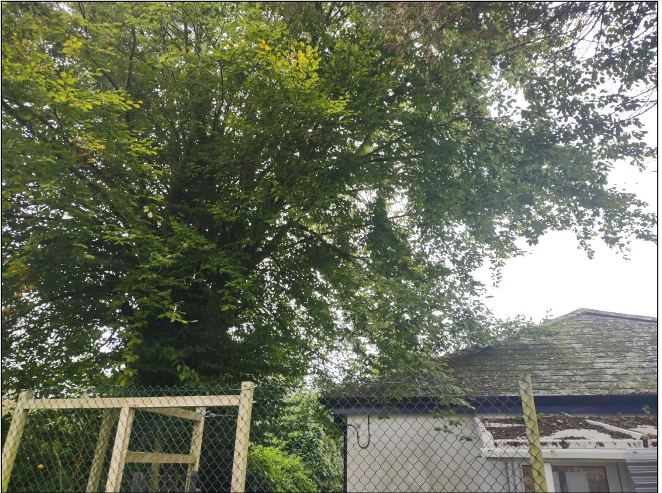
Photograph 1 – Beech T555 rubbing on roof
