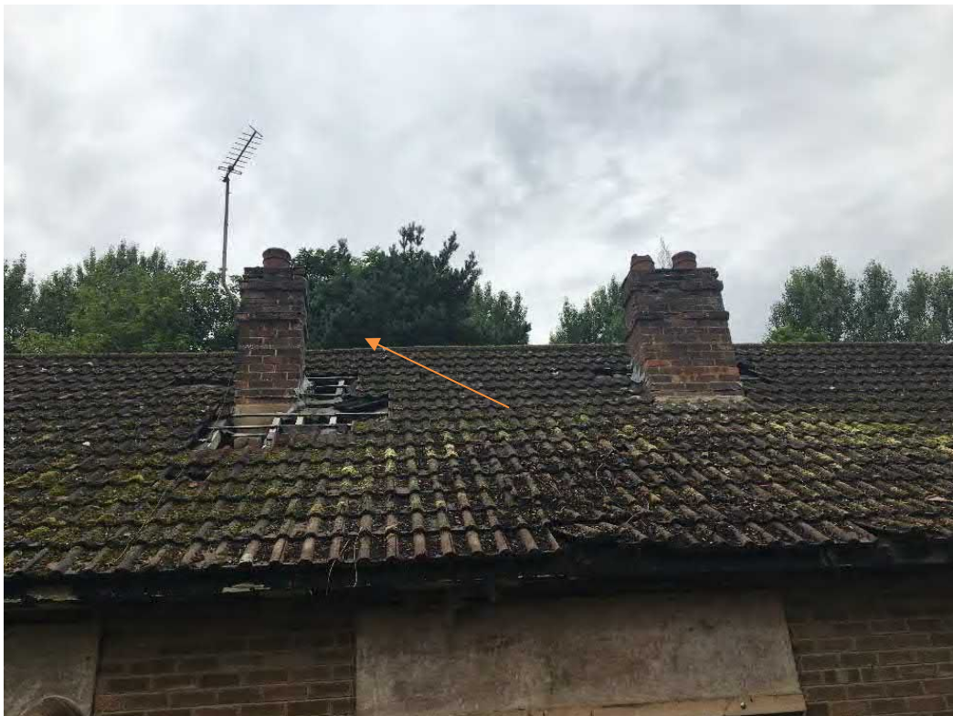
Photograph 6 – Eastern roof elevation of Building 1 with roost access point in roof structure
