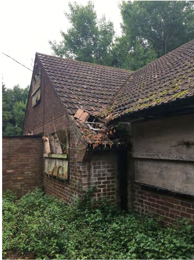
Photograph 7 – Missing roof tiles and warped boarding on Building 1
