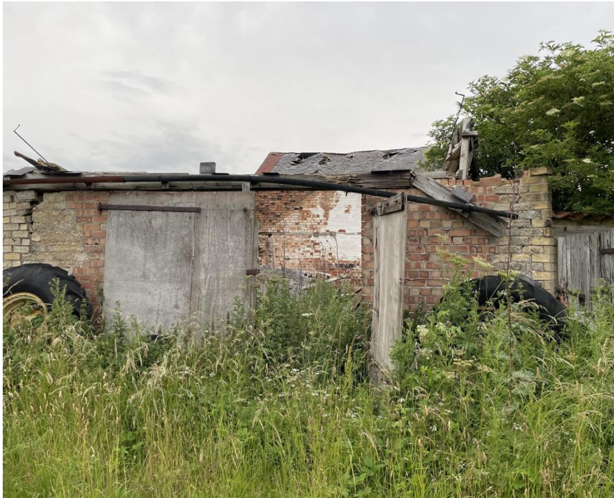
Photograph 13: Collapsed building north side of Building 3
