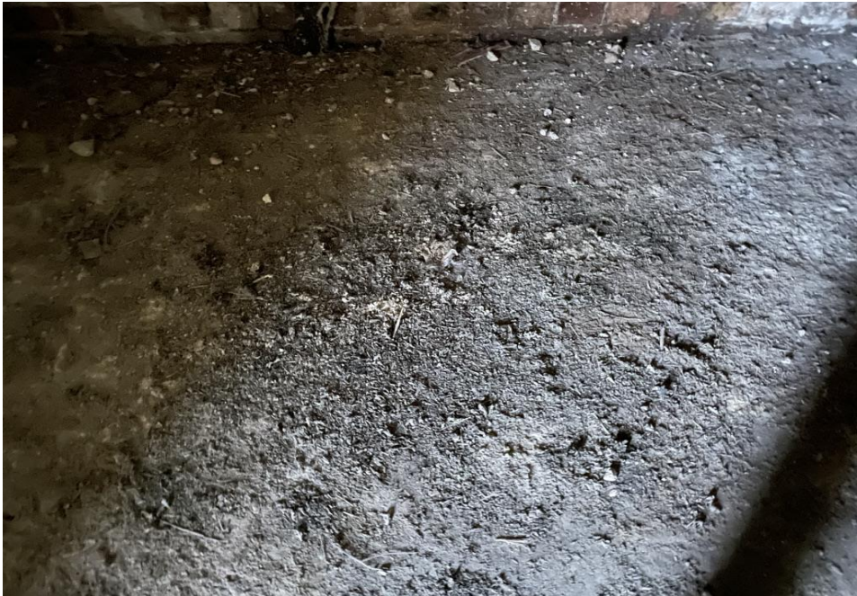
Photograph 25: Degraded barn owl pellets within Building 2
