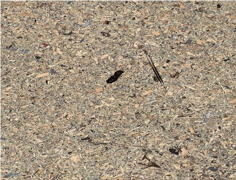
Photograph 18: Bat dropping recorded in Building 2
