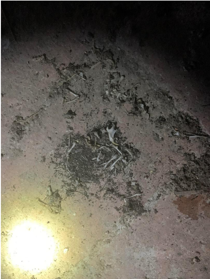
Photograph 26: Degraded barn owl pellets within Building 2
