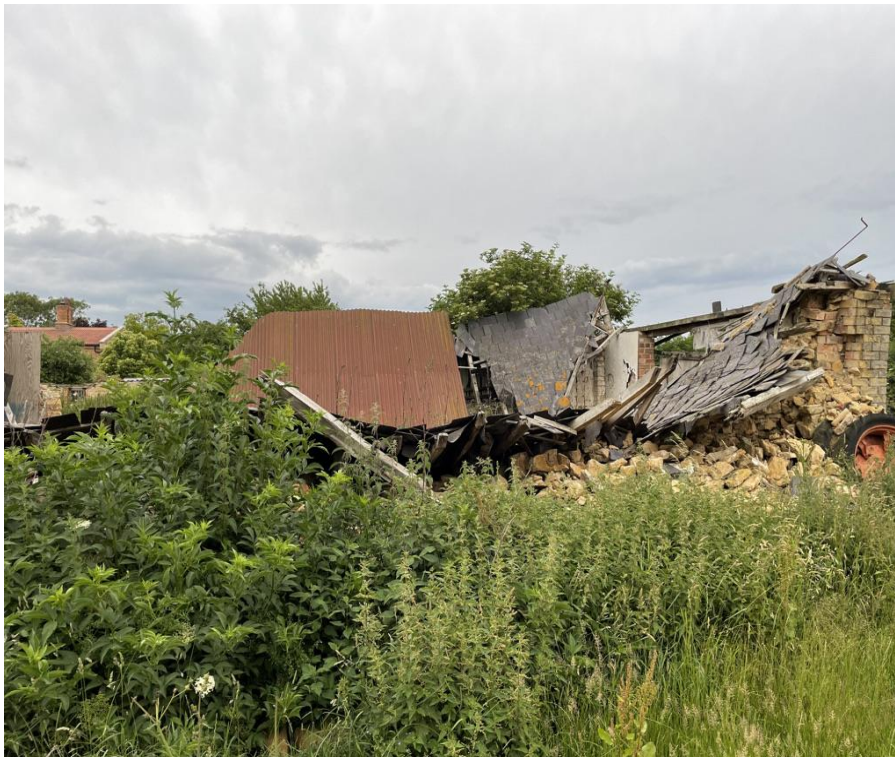
Photograph 12: Collapsed building south side of Building 3
