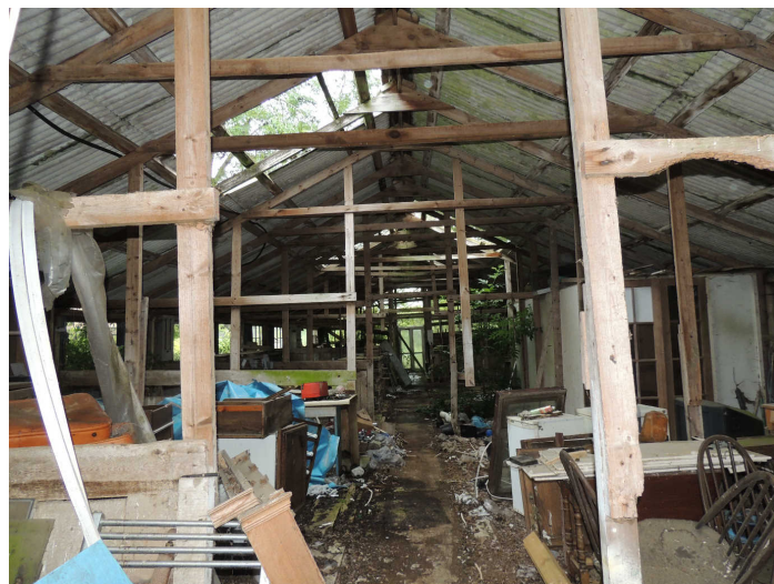
Photo 5: Note gaps in roof
