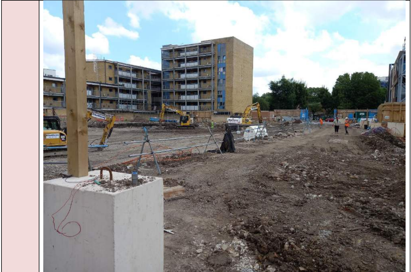
PLATE 4 Campus site, western boundary hoarding being removed to excavate the remaining soils on the banks around the western boundary.
