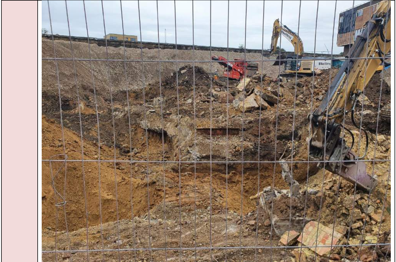
PLATE 3 View looking north west across the RST area which is hosting stockpiles of crushed and screened materials.
