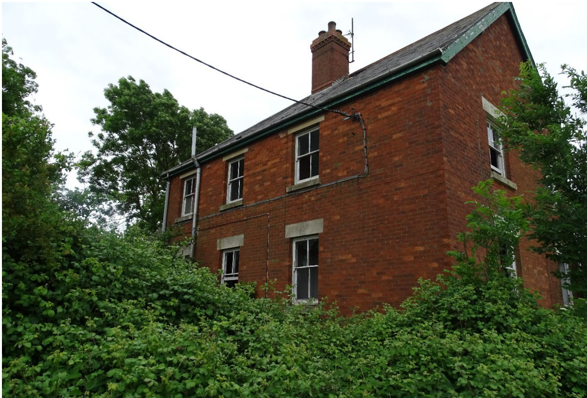
Image 10 – Building one – East facing elevation which has a moderate floor cover of scrub/brambles surrounding
