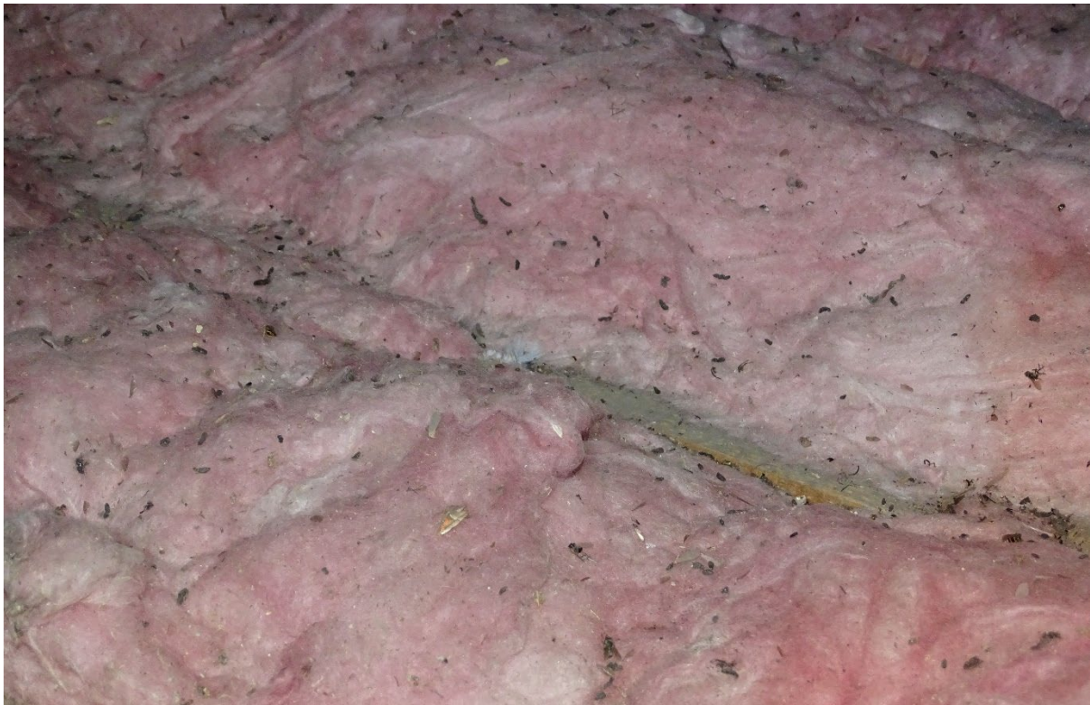
Image 12 – Building one, confirmed bat droppings within the main roof void spaces of the property which has demonstrated activity from bats within
