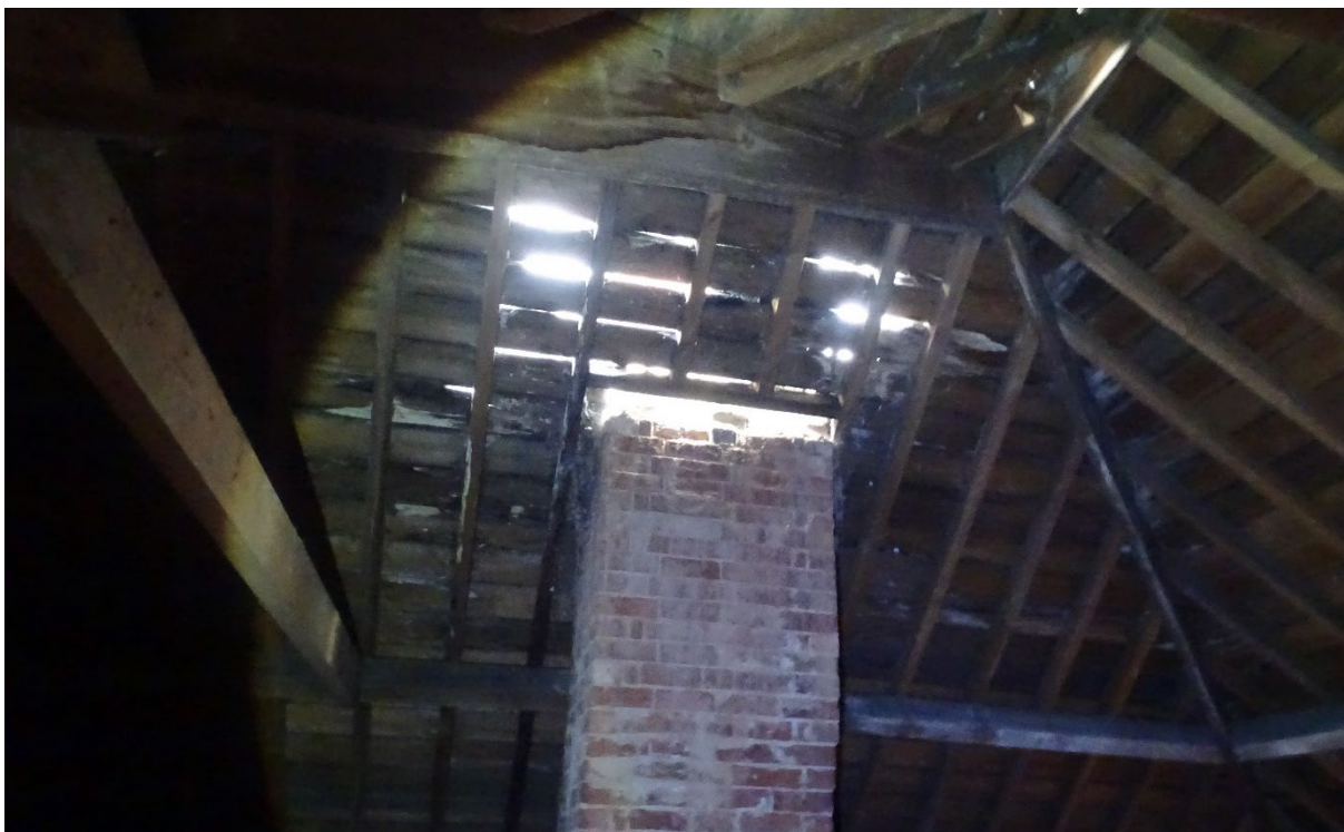
Image 13 – Building one, Internal view from within the main roof void spaces in which a moderate level of natural lighting was observed from several gaps throughout
