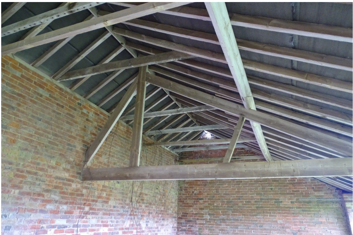
Image 17 – Building three, internal view from within the structure which has demonstrated a felt membrane below the roof coverings with accessible gaps of value to bats
