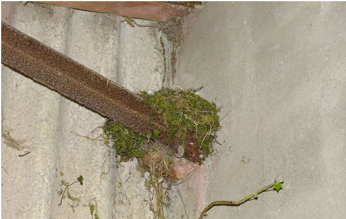
Image 20 – Building four, internal evidence from nesting birds within multiple locations of the structure
