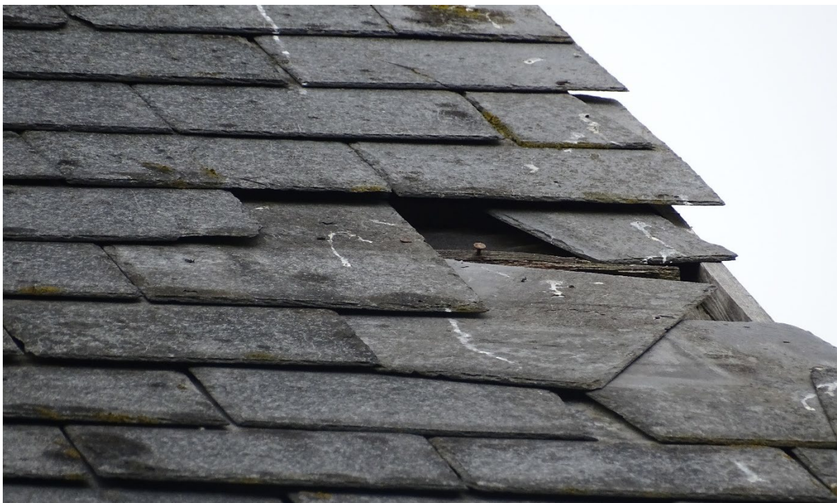
Image 11 – Building one, Moderate level of gaps within the main roof coverings which offer adequate access features for both bats and nesting birds
