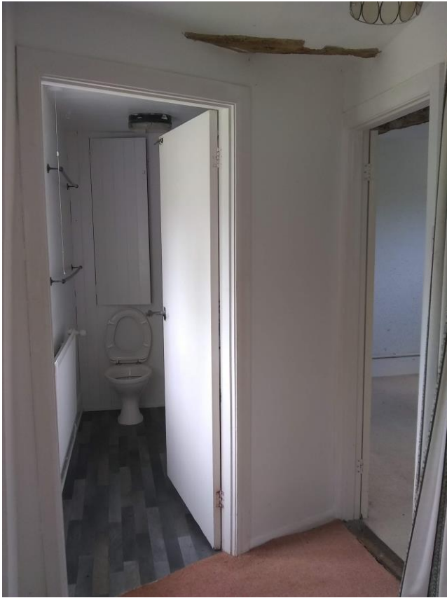
Figure 21: Family bathroom and adjacent bedroom at first floor level. The walls are later plasterboard.
