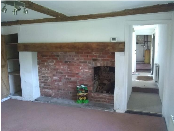
Figure 13: The fireplace in the main sitting room. This appears to have been bricked up at a later date and was likely a large inglenook fireplace
