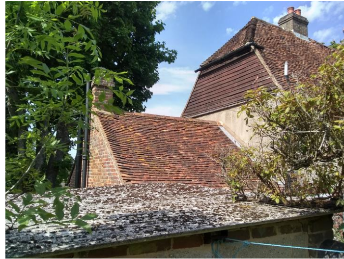
Figure 12: West gable wall with single storey extension and the corrugated roof of the adjacent shed
