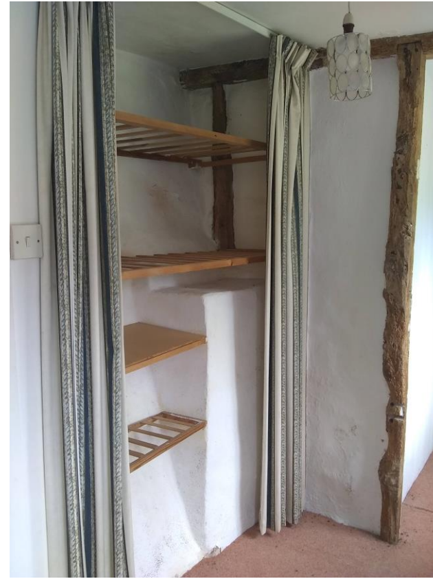
Figure 20: Side of the chimney breast as seen from the first floor hallway
