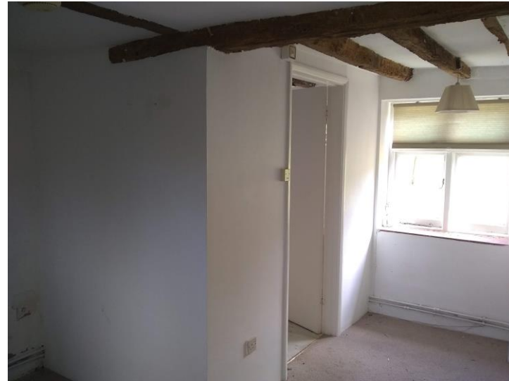
Figure 14: Entrance room at ground floor level with the later plaster board partitions of the WC
