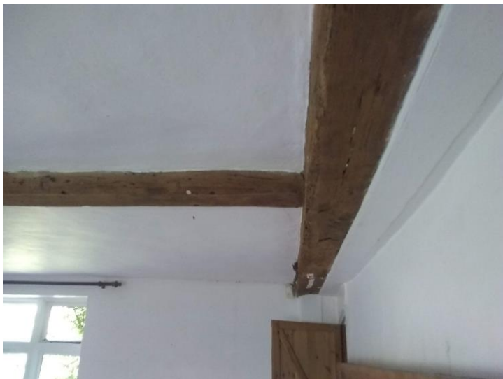
Figure 16: Exposed timber frame beams in the ground floor in the central ground floor room (sitting room)
