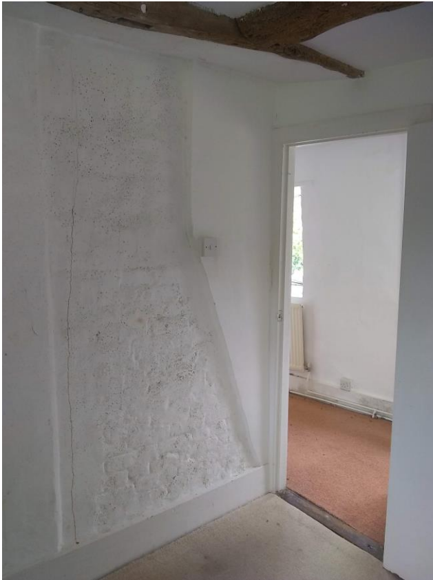
Figure 19: The rear of the chimney breast from downstairs
