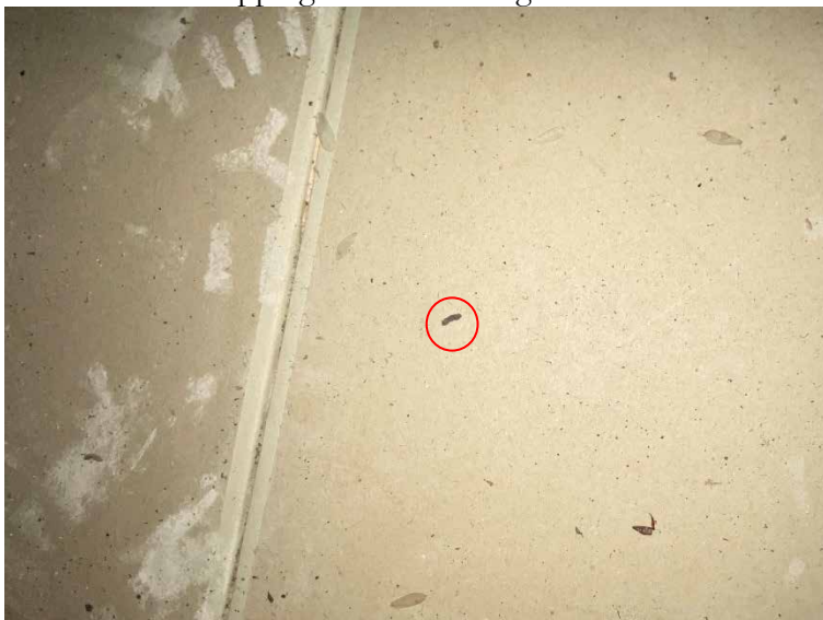
Plate 4 – bat dropping located in the games room roof void.
