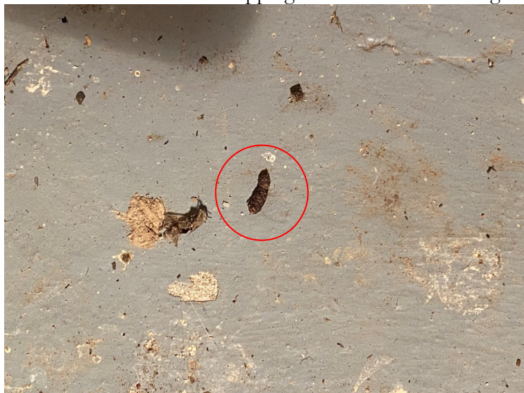
Plate 14 – location of bat droppings below internal south gable.
