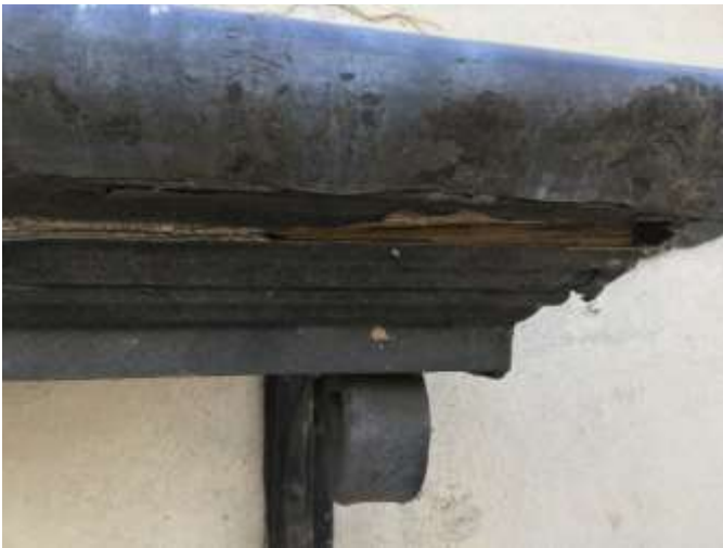
Photograph 5 Damaged timber to flat roof
