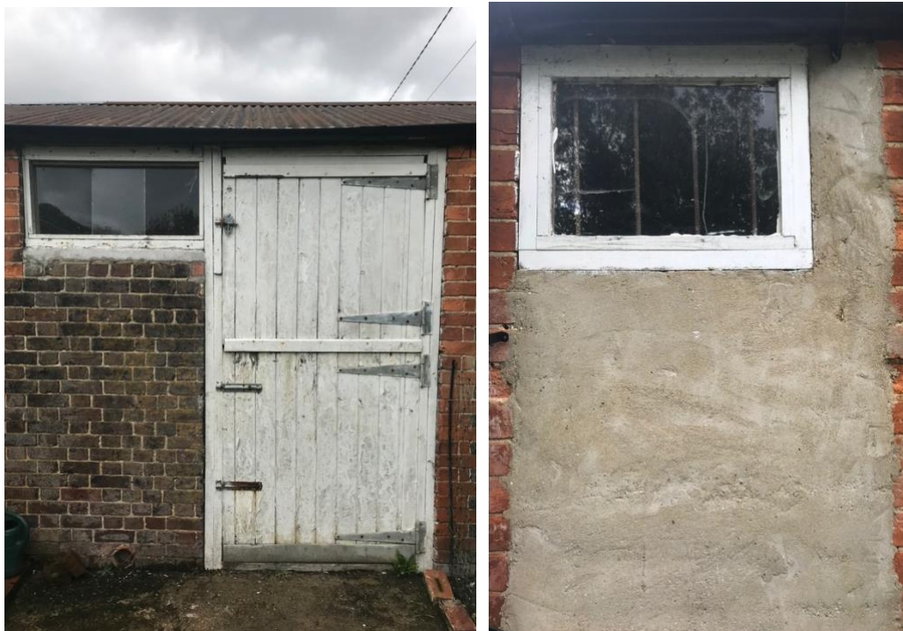
Fig.16: New windows and enlarged doorway to incorporate stable doors in the east block. Blocked up doorway and new window in the east block.
