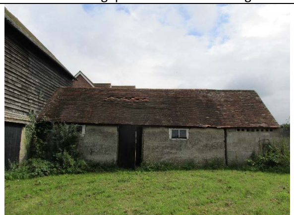
Plate 6: south-western aspect of S2 showing missing roof tiles
