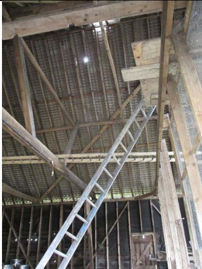
Plate 7: Interior of S1 showing gaps in roof and wooden platform
