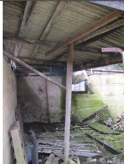
Plate 16: Interior of S3 showing dilapidation
