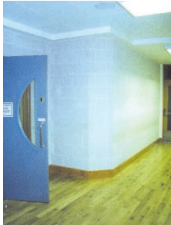
Where doors must swing out into a corridor they should be set in a recess
