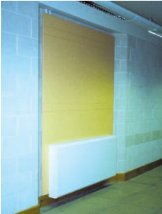
Radiators and other hazards should not project into circulation areas
