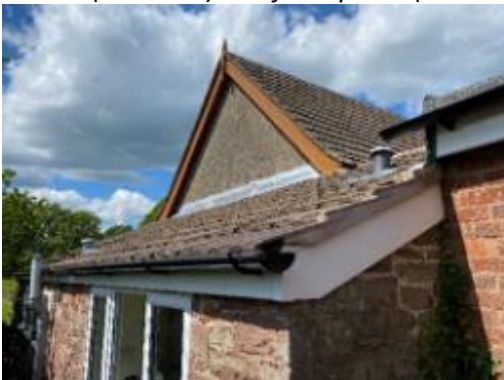
Plate 3: Rear of the Church showing the single storey sloped roof extension from 1893 (section 2) and the joins of sections 1 -3.
