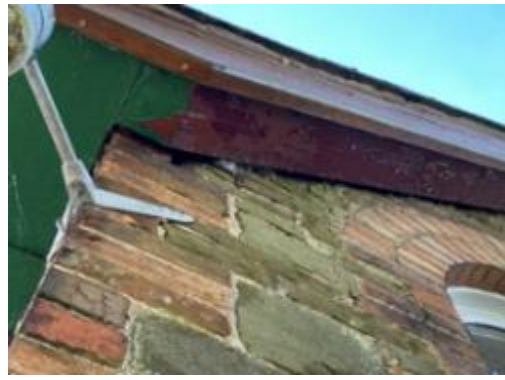
Plate 6: Gaps under the soffits.
