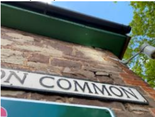
Plate 5: Gaps in the pointing of section 1.
