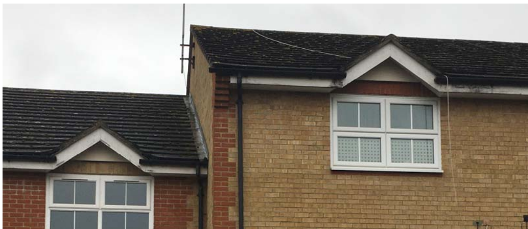
Fig 1, 2 & 3: Rotten balustrade to rear external staircase, defective rainwater goods and rotten fascias and soffits.
