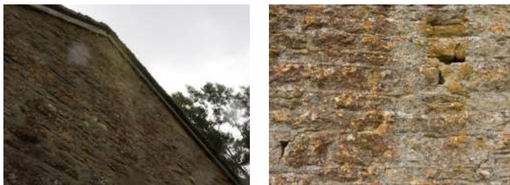
Figs. 7 & 8 Verges (L) and stone wall showing cavities in the pointing (R)
