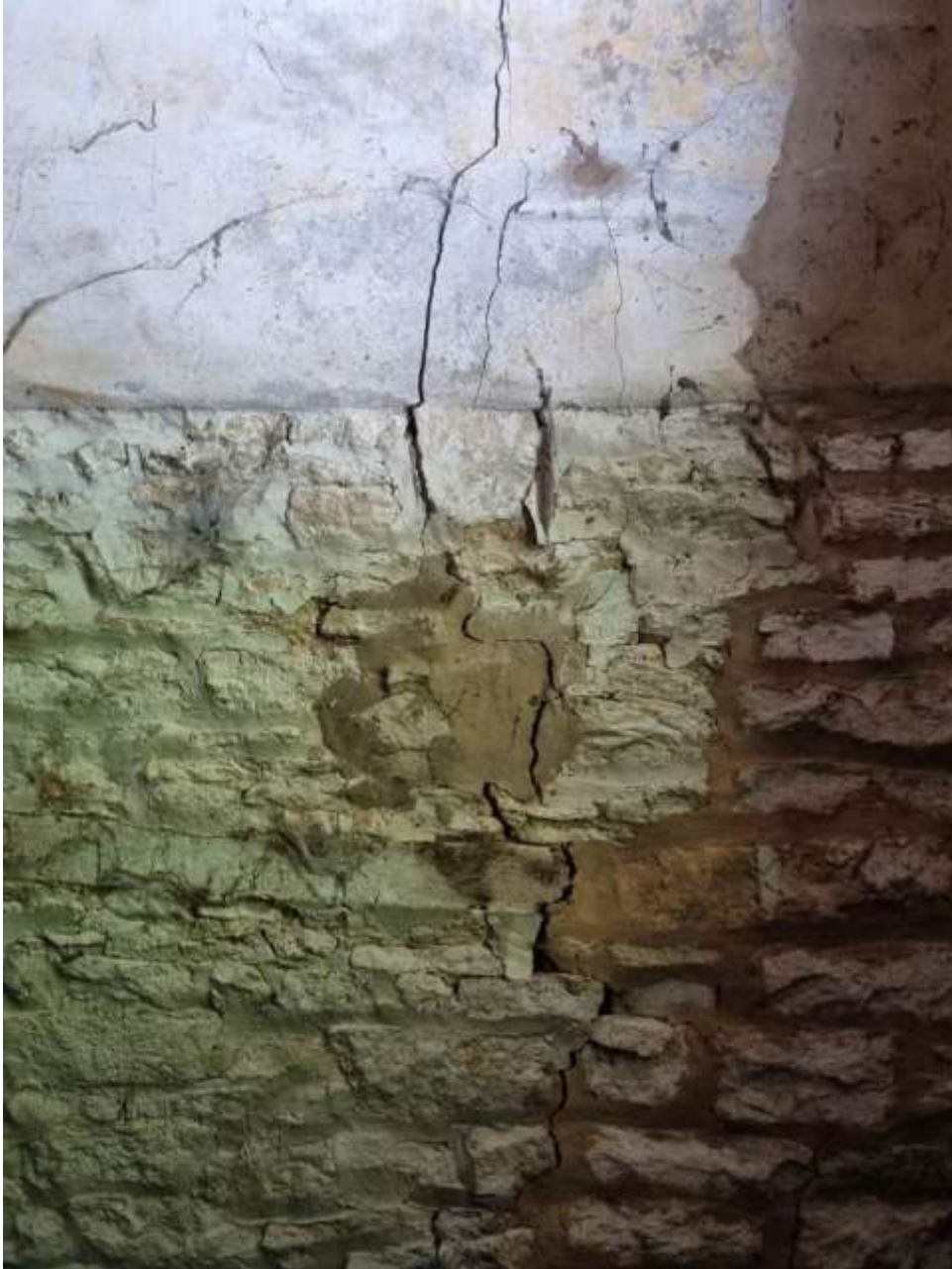
Photograph 6: Showing internal cracking to walls
