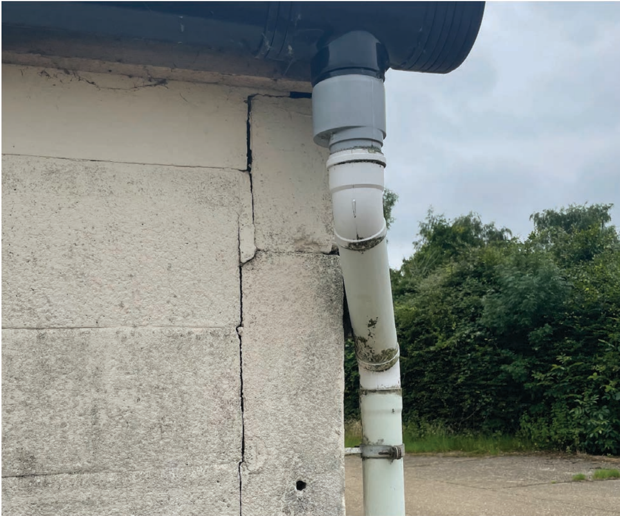
Image 9.0: Vertical cracks at juncture of wall panel abutting end portal frame.
