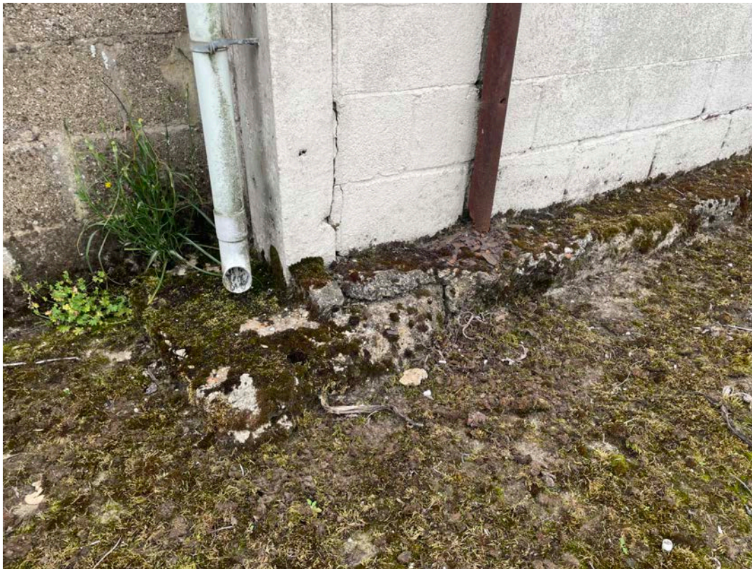
Image 10.0: Excessive SILT to head of concrete slab and moss growing in this medium.
