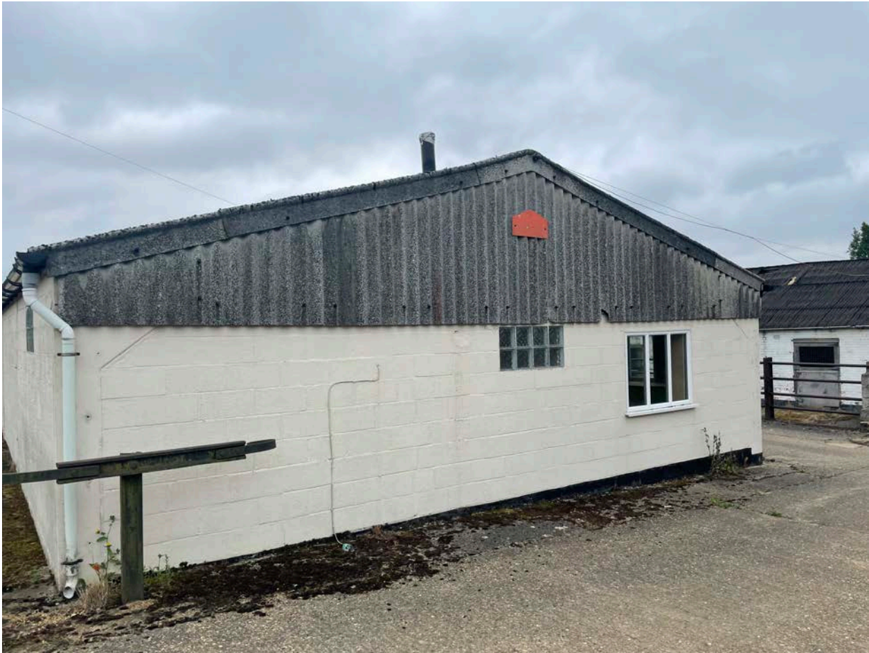
Image 13.0: Stack/ Flue rising through head of roof structure. Note gradual 200mm fall, side to side of the structure.
