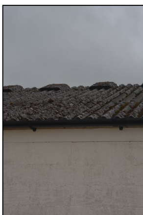
Figure 11 – Gaps between corrugated sheets and ridge
