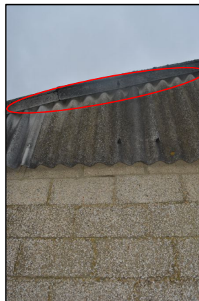
Figure 10 – Gaps where the corrugated asbestos sheets and verge meet on north-west elevation
