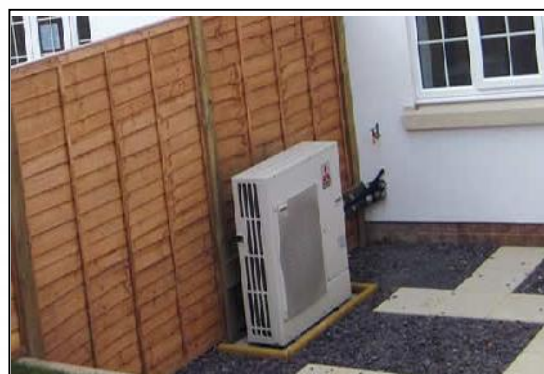
ASHP Installed on a new dwelling
