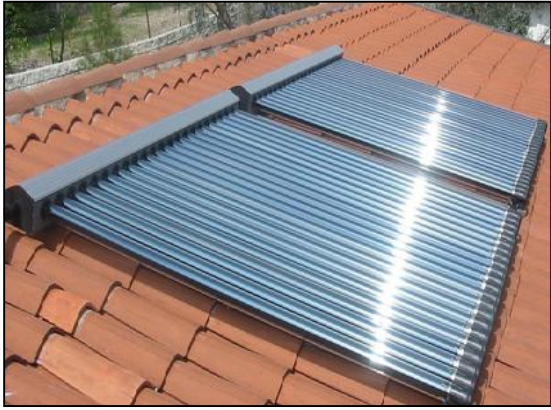
Solar Evacuated Tubes
