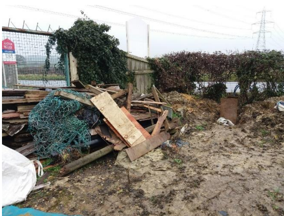
Photo 9 Demolition rubble next to main entrance. Low managed hedge on eastern boundary by road also visible.
