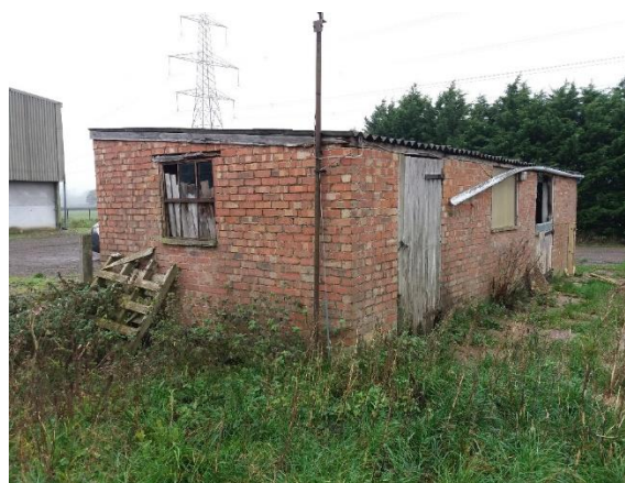
Photo 6 Block 2 brick, corrugated asbestos stable block. Note rotten window frames and collapsing guttering.
