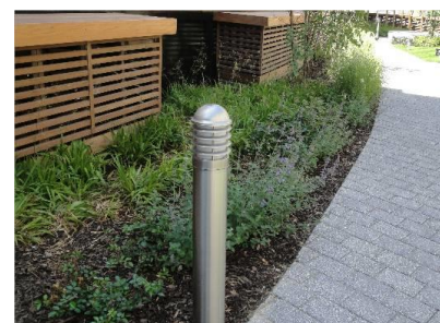
Bollard lighting is bat friendly
