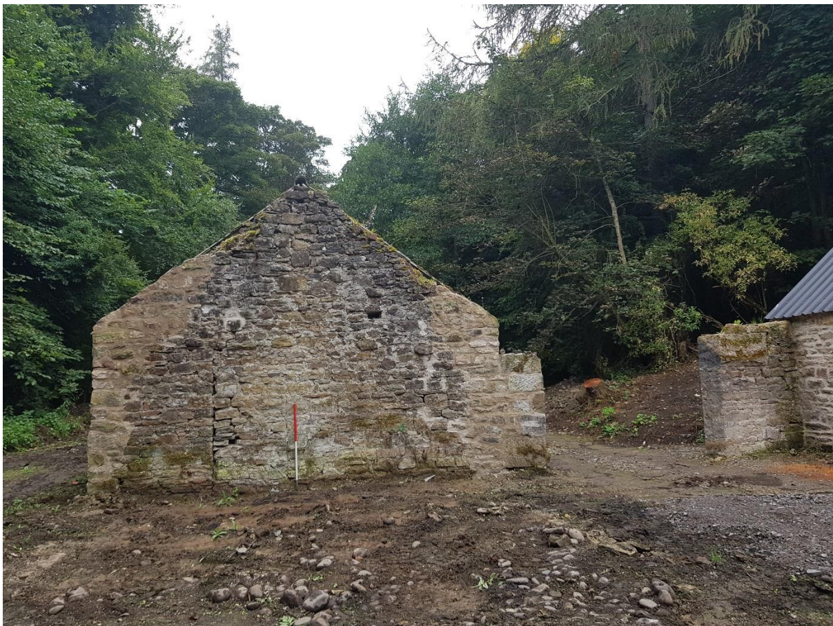
Figure 20. The surviving W gable of the S building. A blocked doorway is located to the left of the ranging pole
