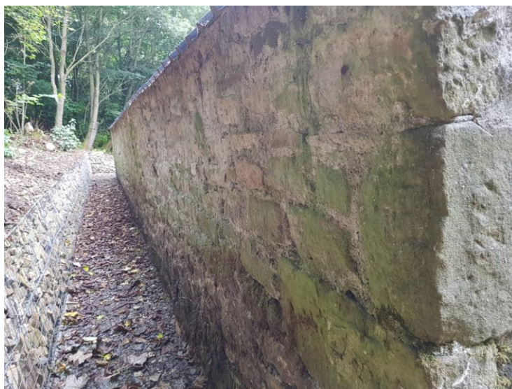
Figure 14. The rear wall of the N building. The earth was cut away from the wall in 2021 to allow it to dry out. It had previously slipped down the bank to cover the bottom four courses.
