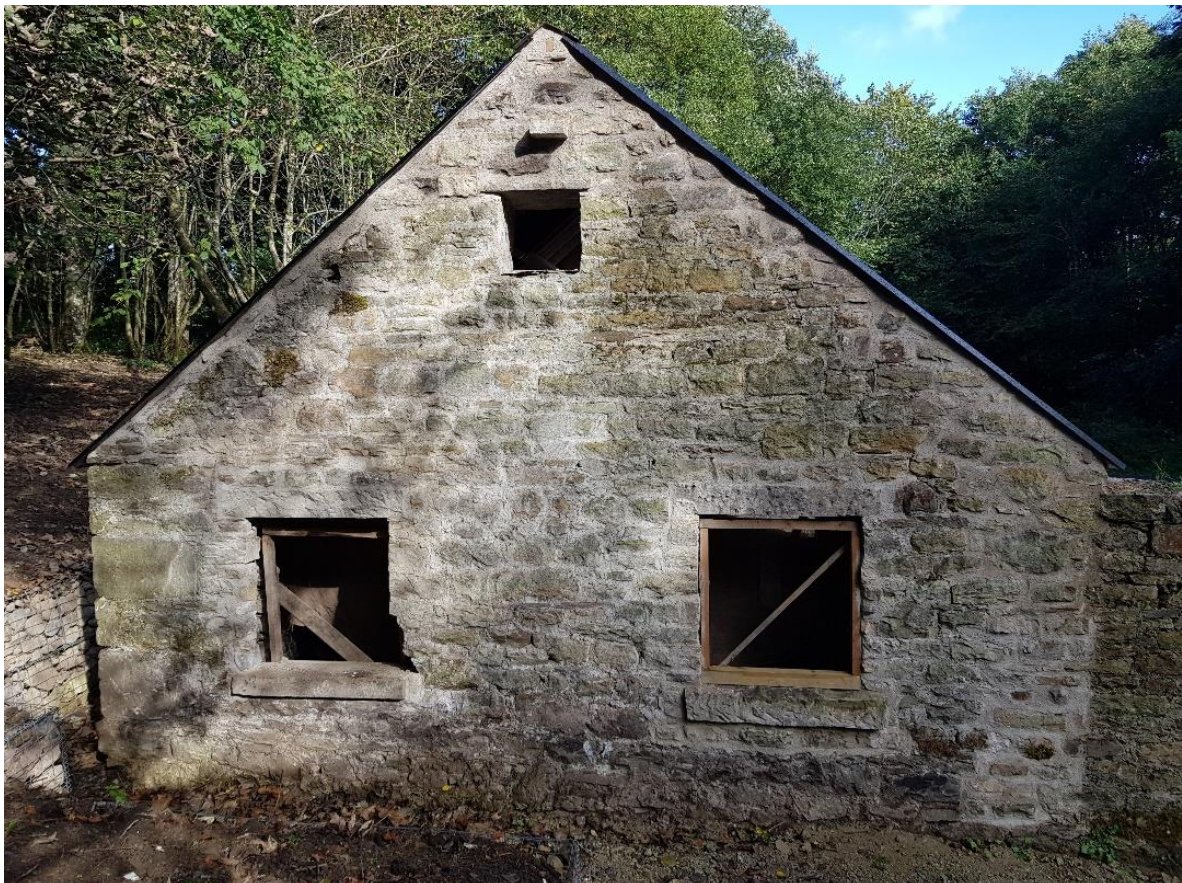
Figure 19. The W gable end in 2021. The repointed whiter area on the right suggests some rebuilding. It is also the location of an adjoining former square building, now demolished.
