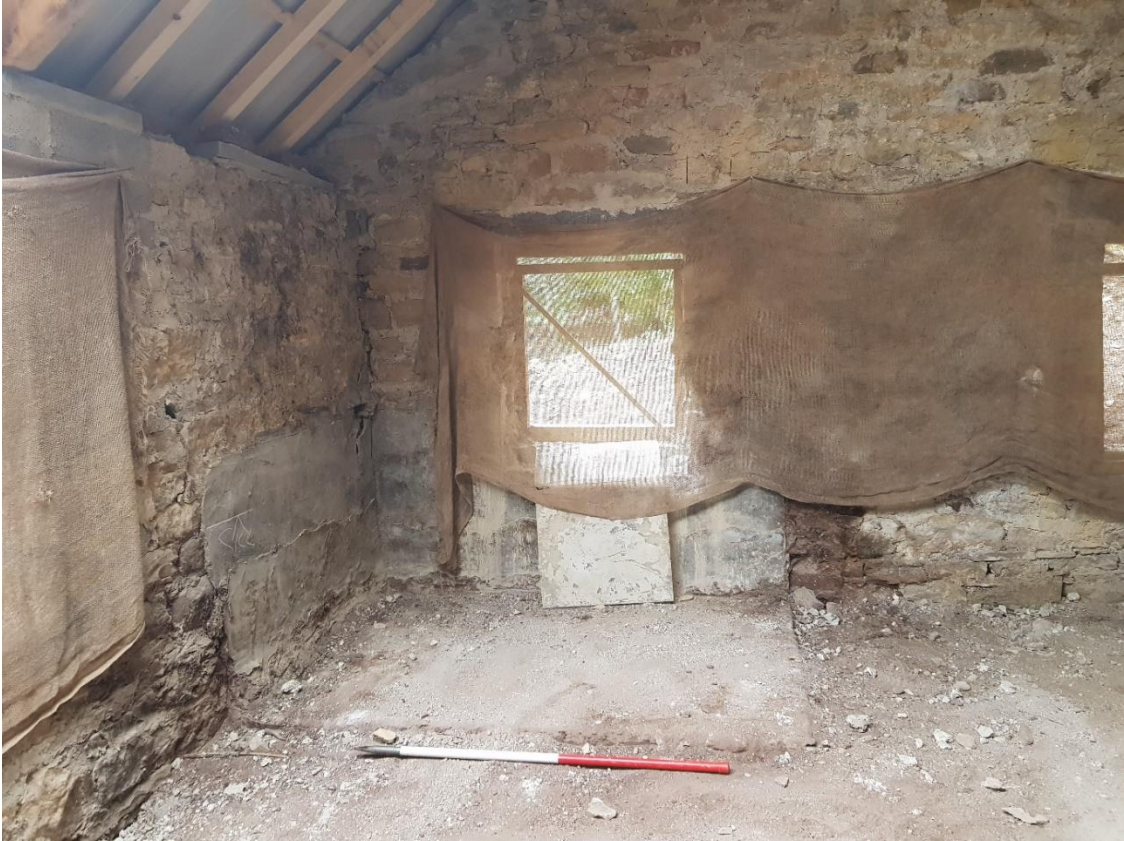
Figure 24. Concrete hardstanding in the SW corner. The window is a modern insertion
