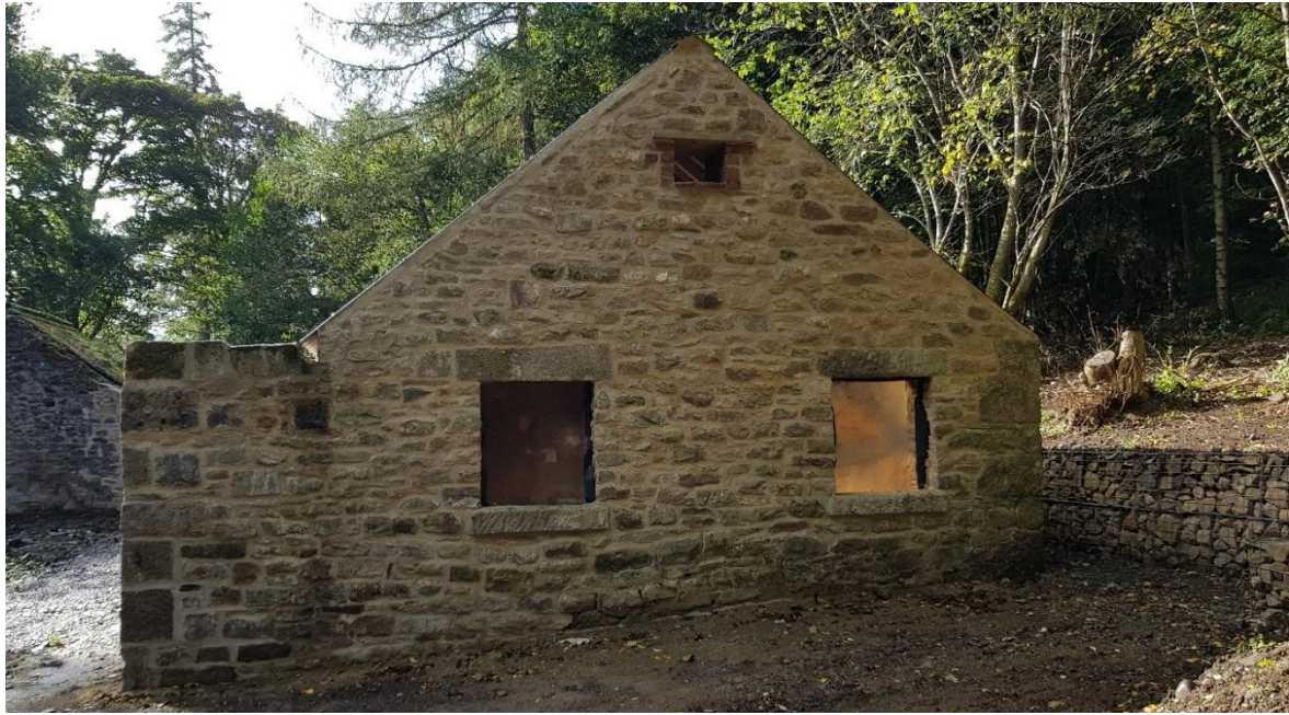
Figure 18. The rebuilt E gable end featuring two square windows and an attic vent opening at the pinnacle of the gable. This elevation was taken down to the bottom five courses and rebuilt in 2021 due to structural issues.
