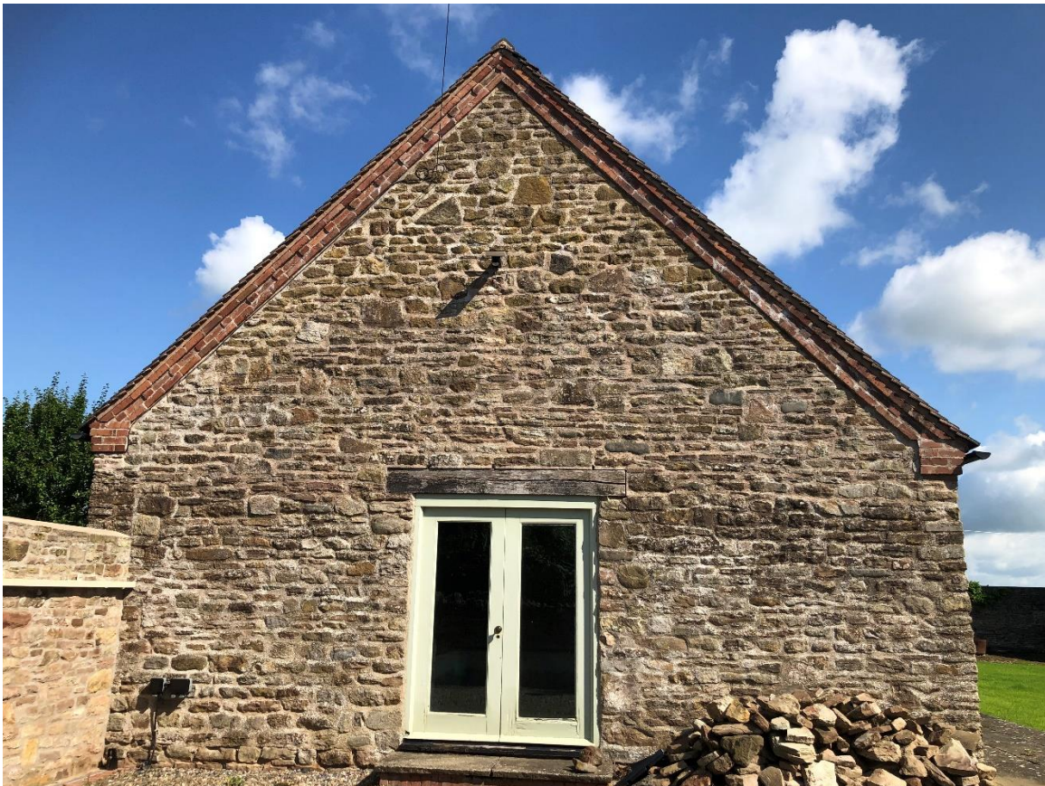
Plate 2. The southern gable end. There are no gaps in mortar at the verges or in masonry; no opportunities for bats are present at this elevation.
