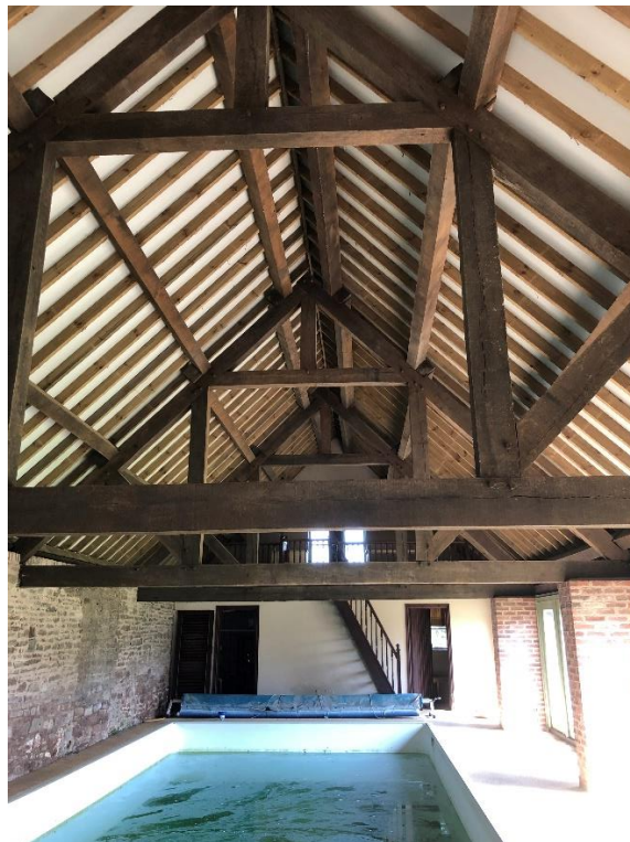
Plate 9. The interior of the pool house, looking towards the northern gable end showing mezzanine floor at the far end.
