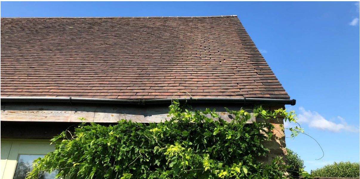
Plate 6. Tiles at the northern end of the eastern elevation are spaced slightly further apart than on the rest of the roof, which may allow access to crevice-dwelling bats to the underside of roof tiles.
