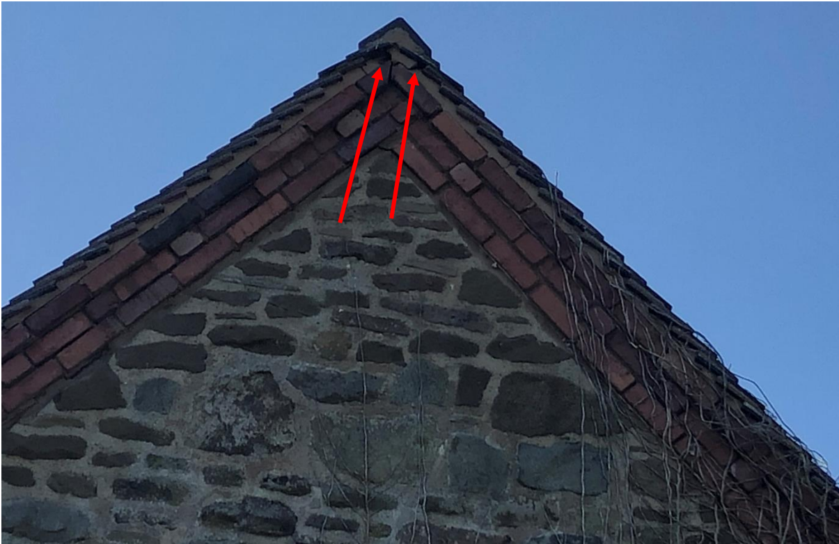
Plate 7. An area of mortar is missing at the apex of the northern gable end, that may allow access to bats to the roof.
