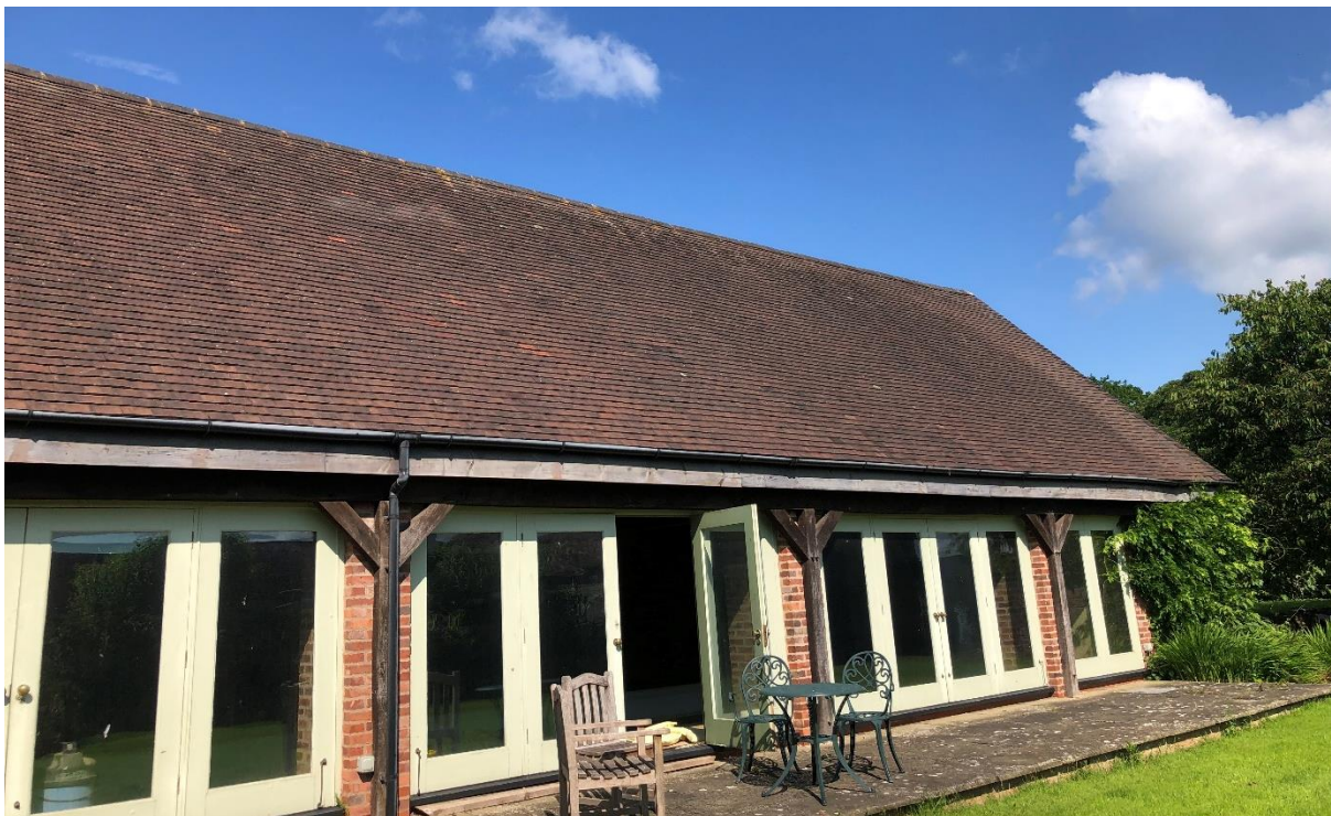
Plate 4. The eastern elevation of the pool house, showing the line of glazed doors and good condition of roof.
