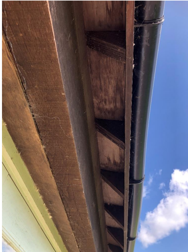
Plate 3. Eaves and soffits are tightly-fitting and well sealed, offering no opportunities for bats.
