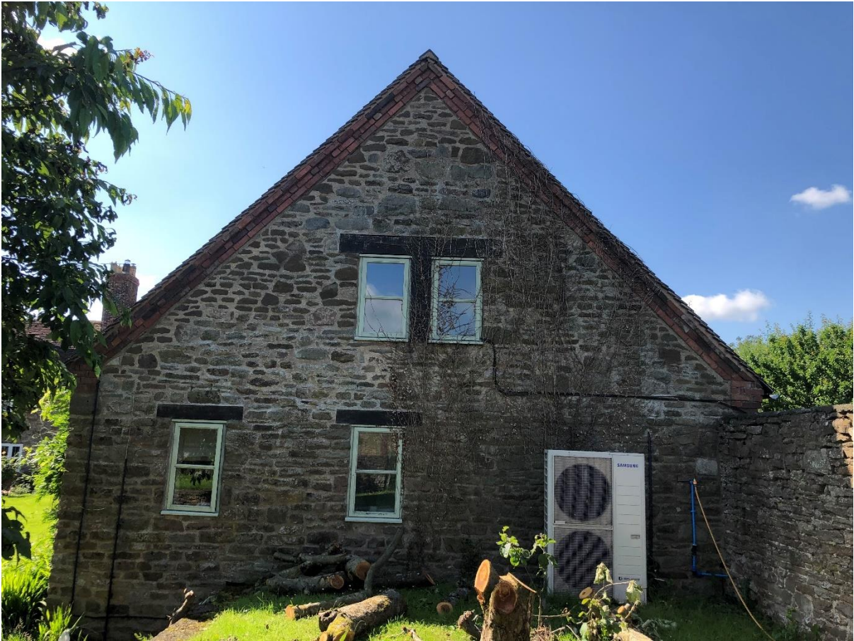
Plate 5. The northern gable end, showing glazed windows and stone work in good condition. There is one small area of missing mortar at the apex of this elevation.
