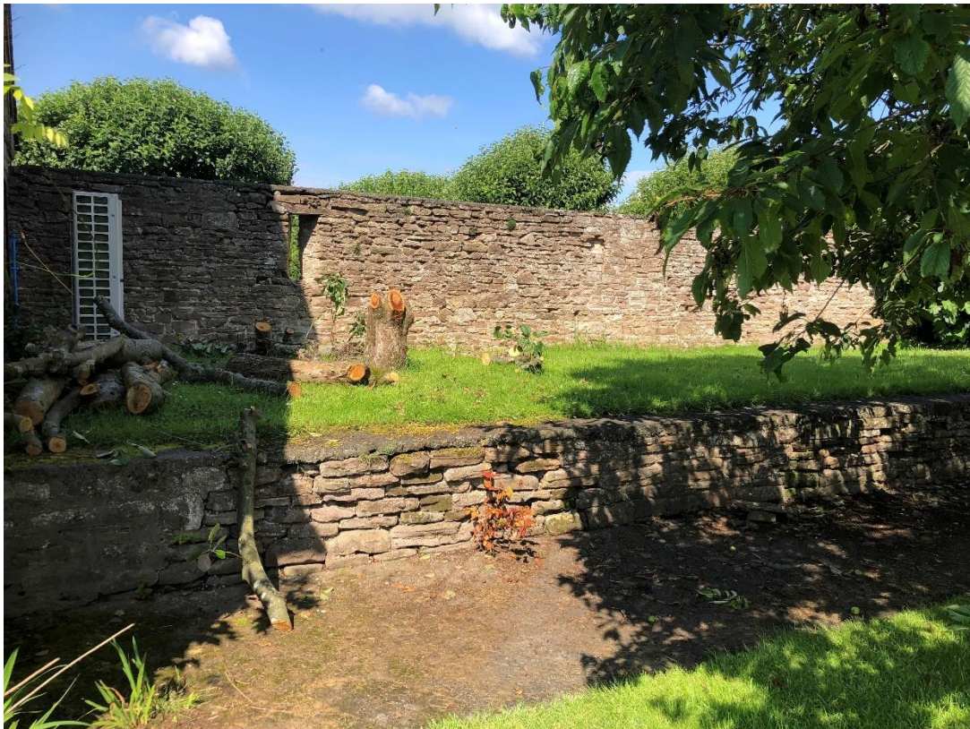
Plate 15. The area proposed for the new extension. It is likely that all or part of the stone retaining wall seen here will be removed to accommodate the proposals. Gaps are present within the wall which may provide suitable terrestrial habitat for great crested newt if present nearby.
