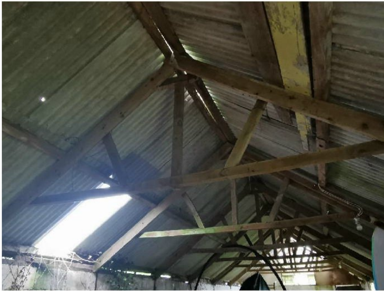
Photo 7: The roof internally. There are large gaps between the wall tops and roof, missing asbestos sheeting and a partly missing roof at the western end.
