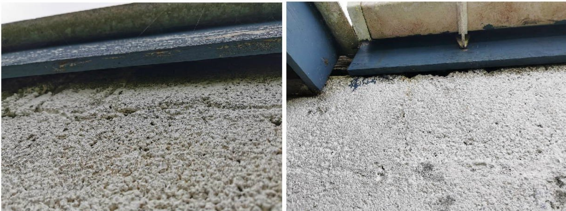
Photo 5, 6: Gaps behind the fascia boarding along the northern extension (left) and part of the northern aspect of the main barn (right).
