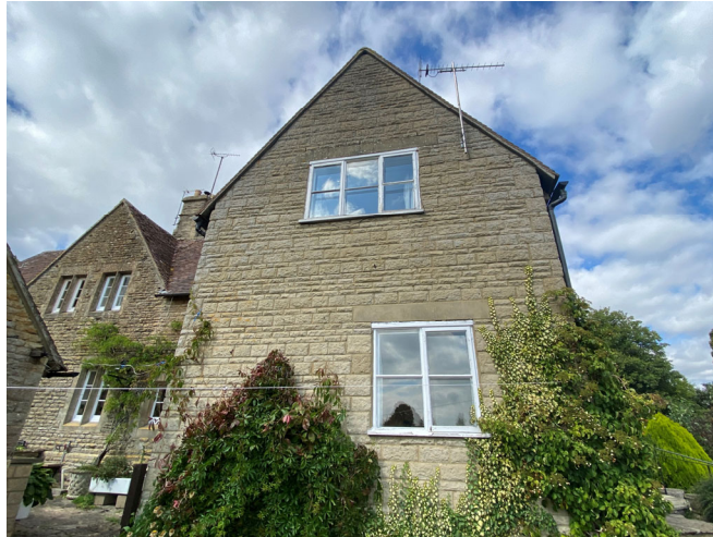
Existing south elevation - Poor quality reconstituted stone and timber storm casements.
