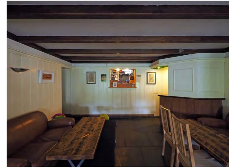
Fig 27: Dining Room from SW: wall with hatch may contain many features of interest behind panelling
