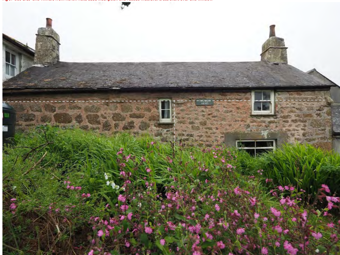
Fig 10: Tinners rear wall annotated to show original probable eaves level with kneeler stone at far right; walling left of central former stair window has larger stones probably due to re-facing or rebuilding; C20 inserted window at far right
