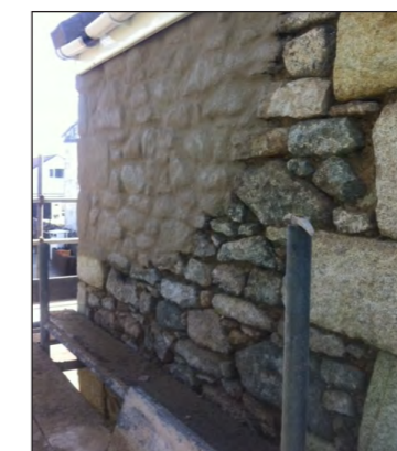
Example of Lime mortar bag-rubbed render to be utilised on interior face of external walls.
