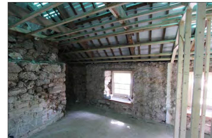
Fig. 19. Poor quality masonry to 1st floor.
