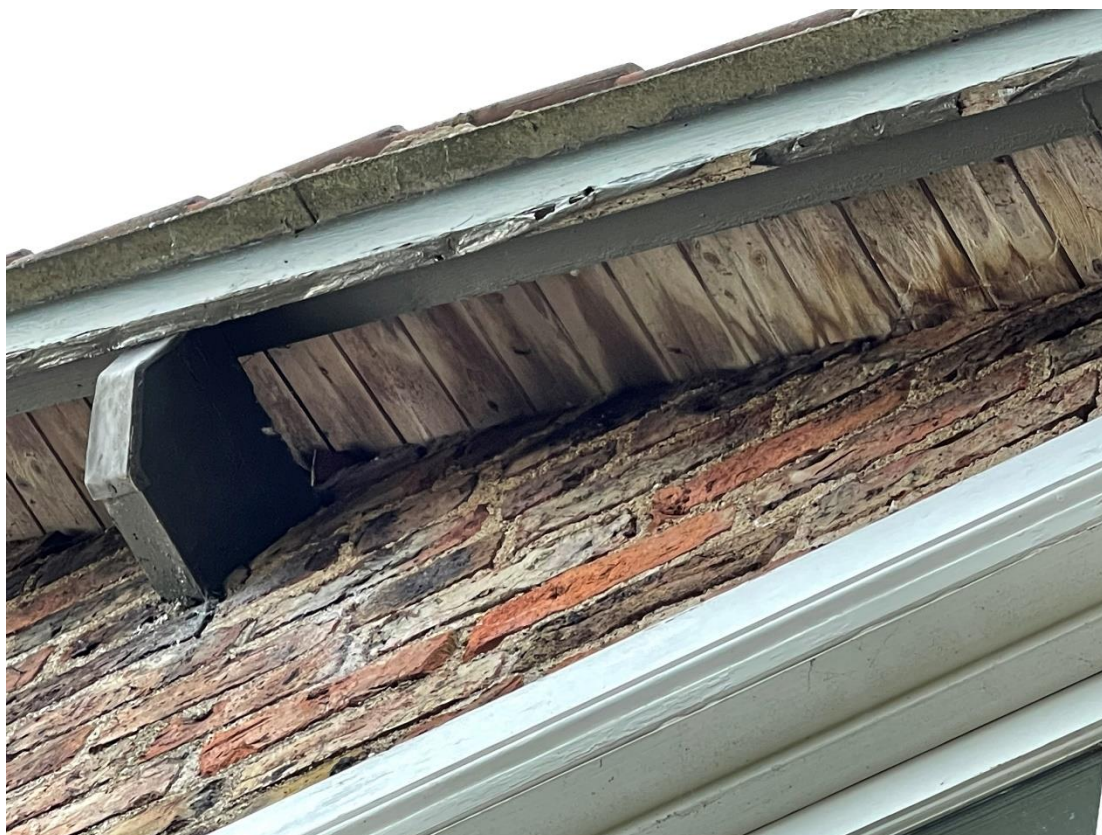
2. Closely fitting soffits, fascias and windows offering negligible roosting potential.
