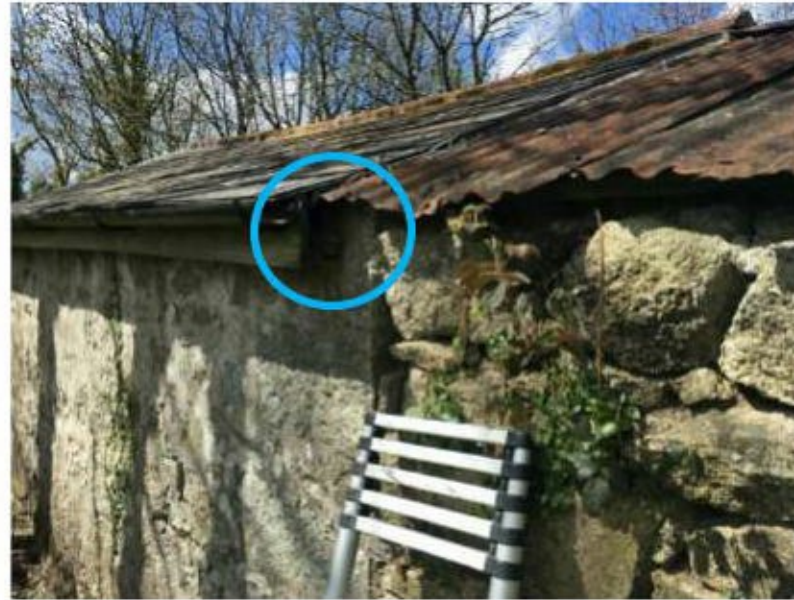
Photograph 4. Broken soffit box and potential bat access.
