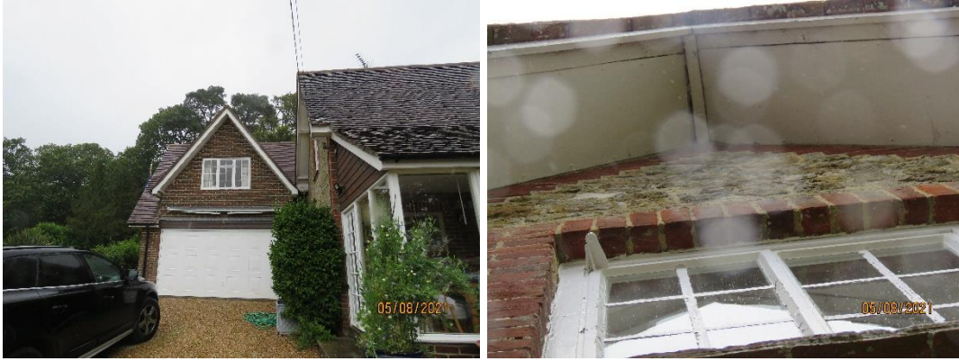
Figures 9 & 10. Showing northwest wing (roof void not affected by proposals) and stone built western elevation gable end of original house where a proposed single storey extension will be located. Also, apex of stone-built gable end with a gap to soffit that may be an access point for the resident bats.
