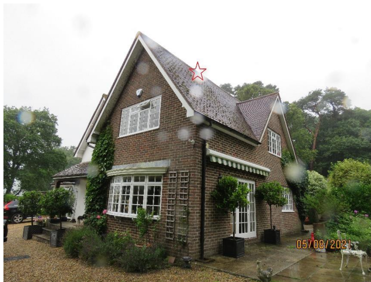
Figure 8. Showing east wing built in 1978/79. The red star indicates approximate position of maternity cluster in roof void.
