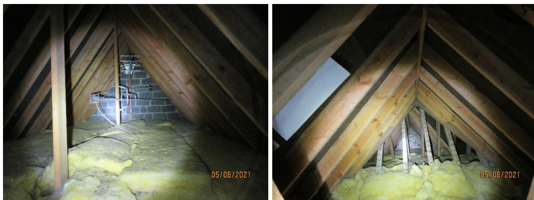
Figures 4 & 5. Main roof void. Numerous bat droppings were scattered on the roof insulation and a small maternity cluster of Brown Long-eared bats was observed at the ridge. Figure 5 is looking west along an inaccessible part of the void above the main body of the house towards a stone-built gable end.
