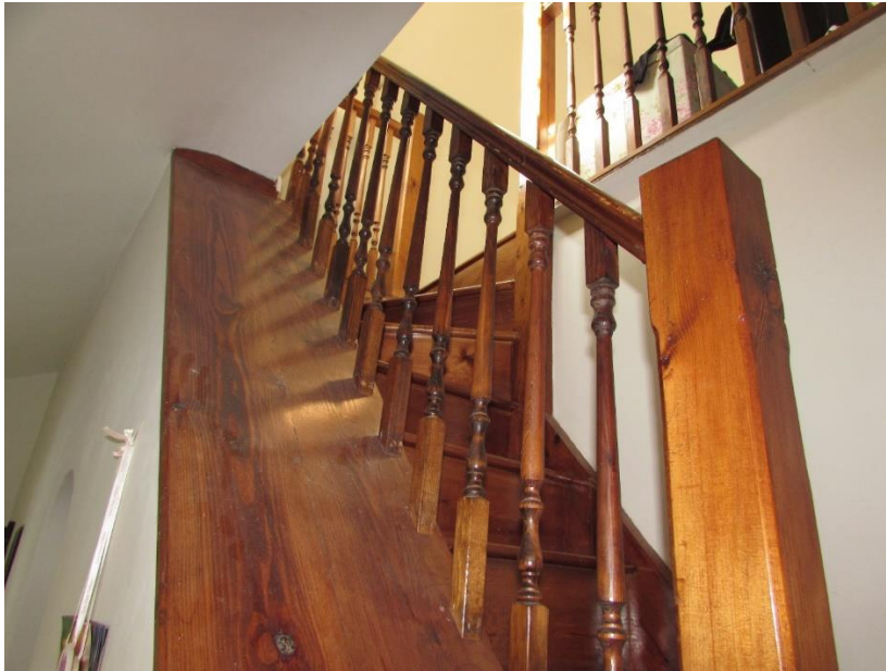
Figure 1 - narrow steep staircase
