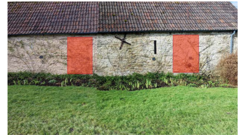
Potential Previous Openings on East side of current office to previous barn/ structure - Now infilled with masonry
