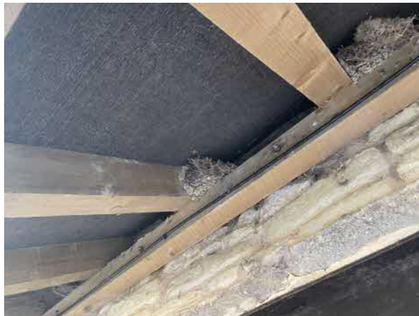
Photograph 17: Swallow nests under the canopy above the garage doors.
