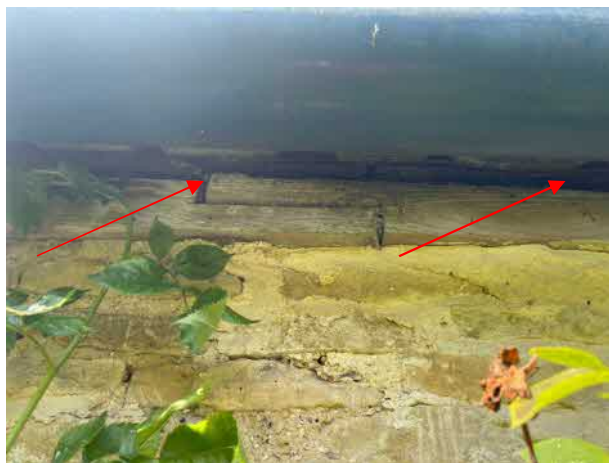
Photograph 16: Annex – gaps in the eaves.
