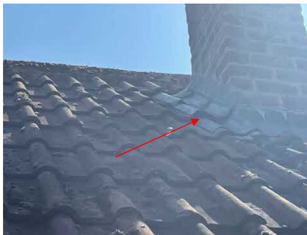
Photograph 13: Annex – gaps under tiles.
