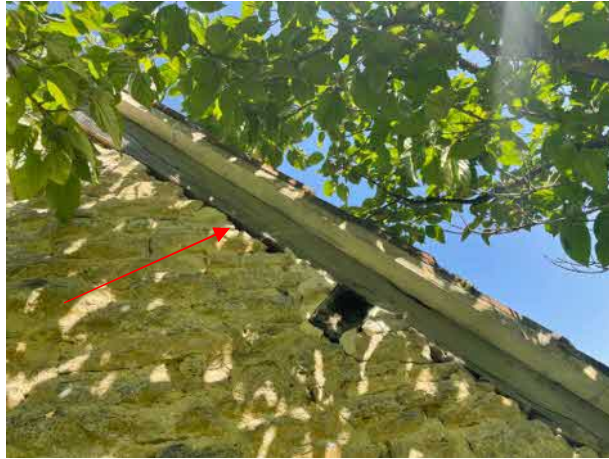
Photograph 15: Annex – Gaps on the south gable roof verge.
