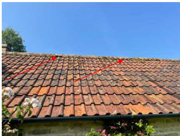
Photograph 14: Annex – gaps under ridge tiles – vent left (meshed) missing mortar right.
