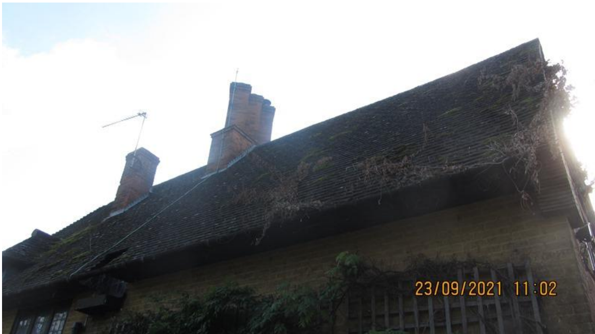
Photo 6. Lifted tiles and poor state of roof
