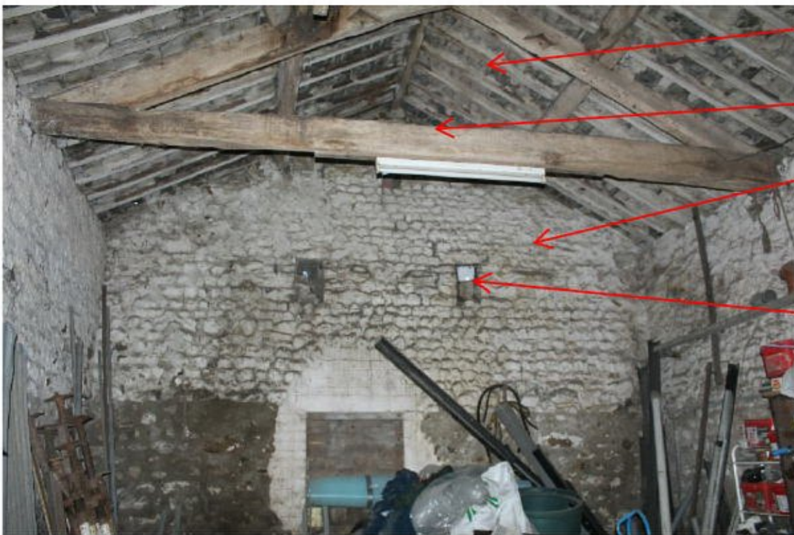
Unlined roof Roof timbers in good condition Walls sealed Ventilation holes partially blocked
