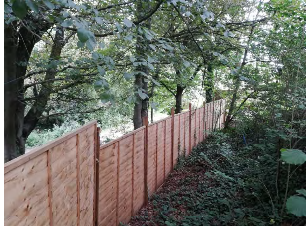
16. Fence towards NE site boundary, preventing access to the bungalows from Tape Lane.
