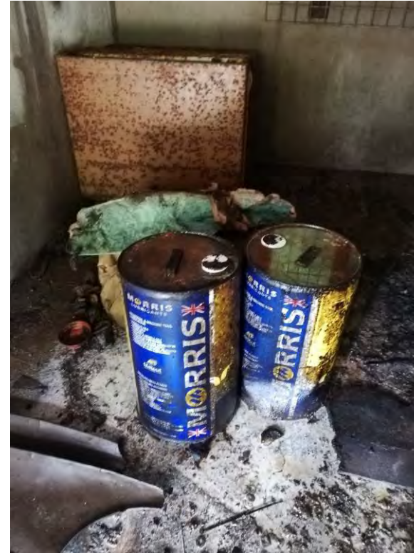
26. Lubricating oil drums inside workshop. Minimal staining and hydrocarbon odour inside workshop, concrete slab floor appears intact.
