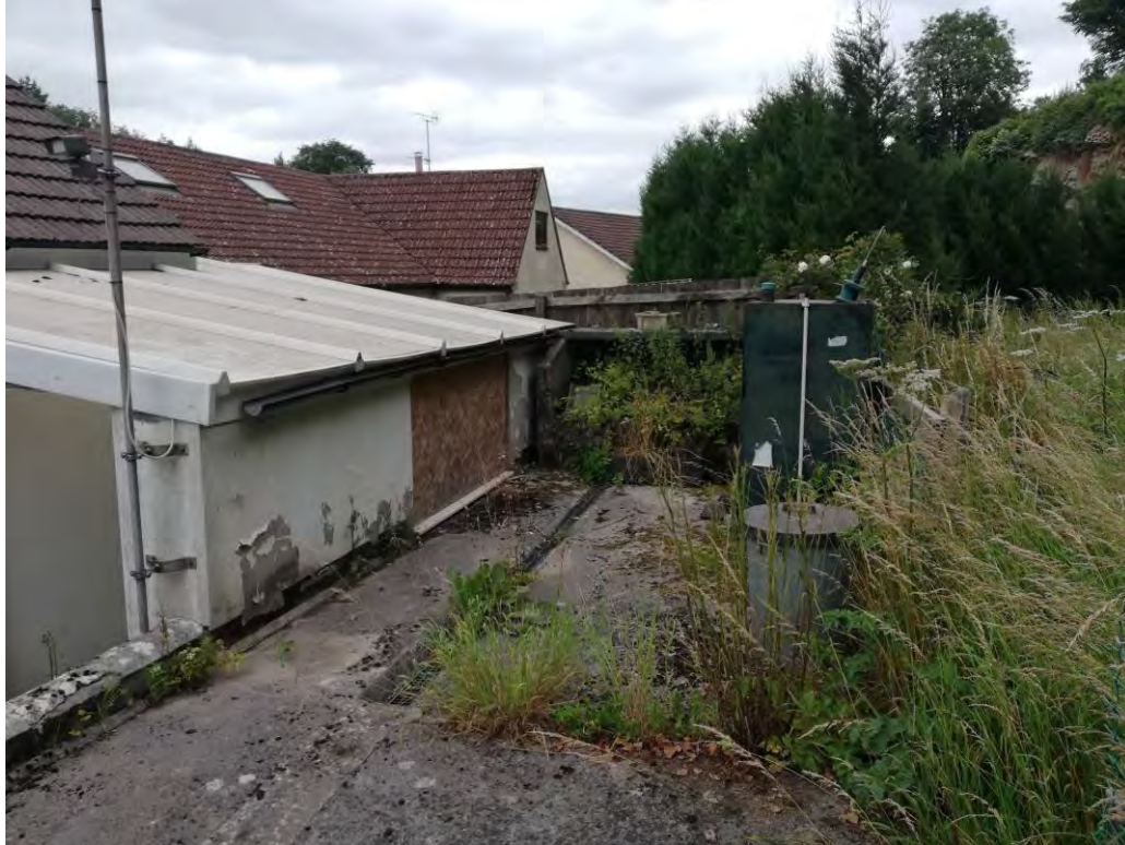
5. Rear of 'Alwyn' (bungalow on E side) indicating location of heating oil tank, looking E.
