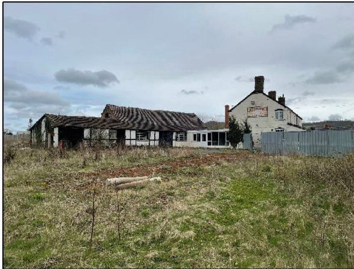
Plate 3. The southern aspect of the Outbuilding and single storey extension (looking north-east)
