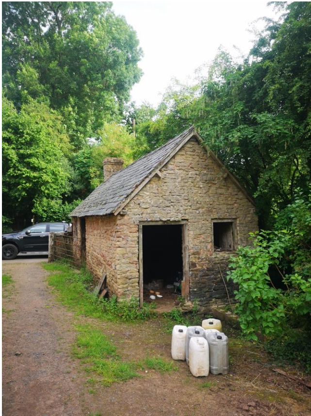
Figure 8 – northern aspect of B3 showing gaps along the gable end
