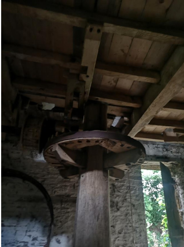
Figure 7 – Internal mill feature with exposed timbers with suitable roosting opportunities for bats
