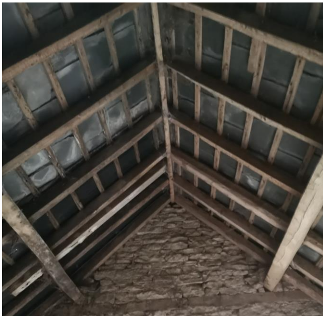
Figure 9 – internal picture of northern gable end with gaps in mortar.
