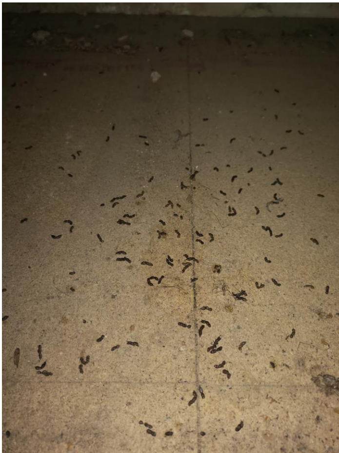
Figure 5 – B1 first floor bedroom with droppings noted on floor
