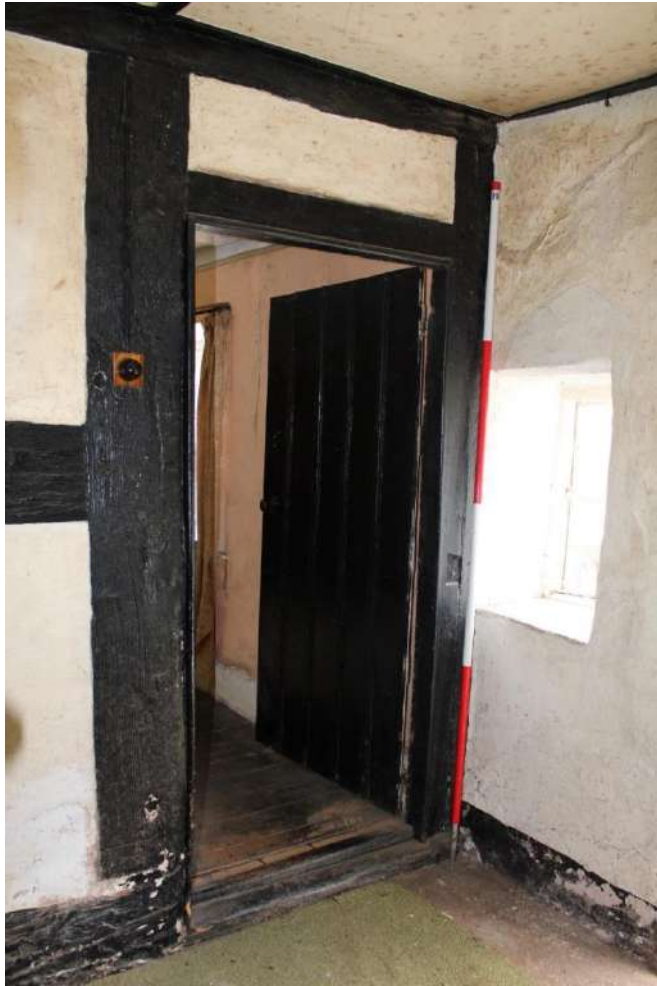
Photo 22: View south along central passageway to door to southern ground floor room
