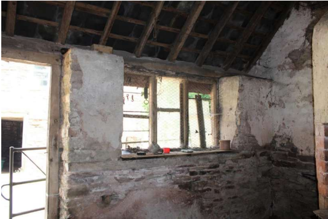
Photo 45: View east through southern room of the Bakehouse with oven just visible to right
