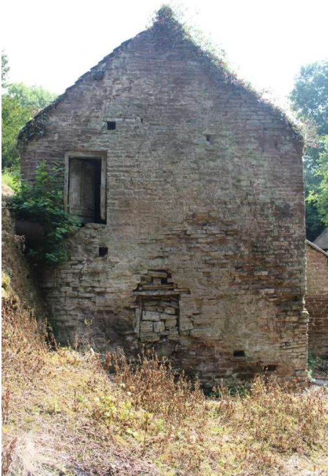
Photo 9: Northwestern elevation of Mill, with metal pipe to left for water to left and mill wheel housing and axle located in the central infilled part of wall
