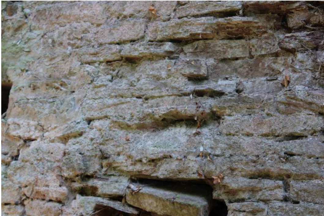
Photo 11: Scarring on wall of Mill from the wheel
