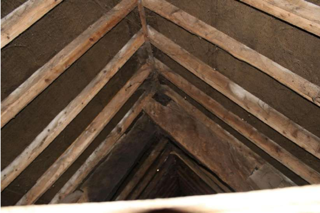
Photo 28: View southeast along roof space (from loft hatch) showing simple roof with truss visible
