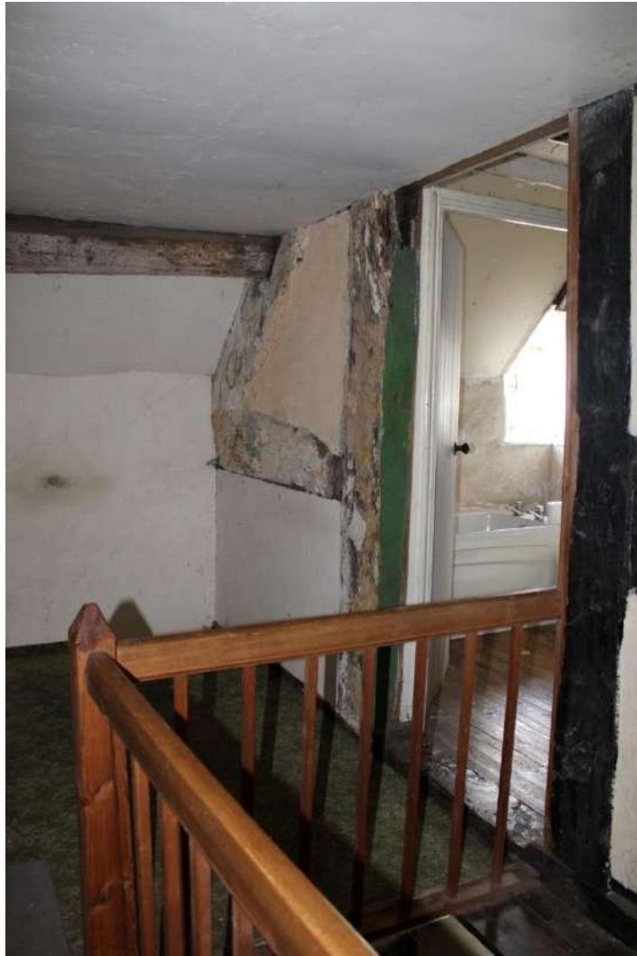
Photo 24: View east across first floor landing to corridor to southern bedroom and bathroom
