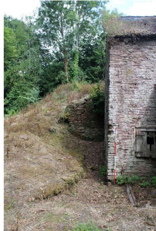
Photo 8: View northeast along northern edge of Mill building to wheel pit and stone lined channel exiting towards Clee Brook
