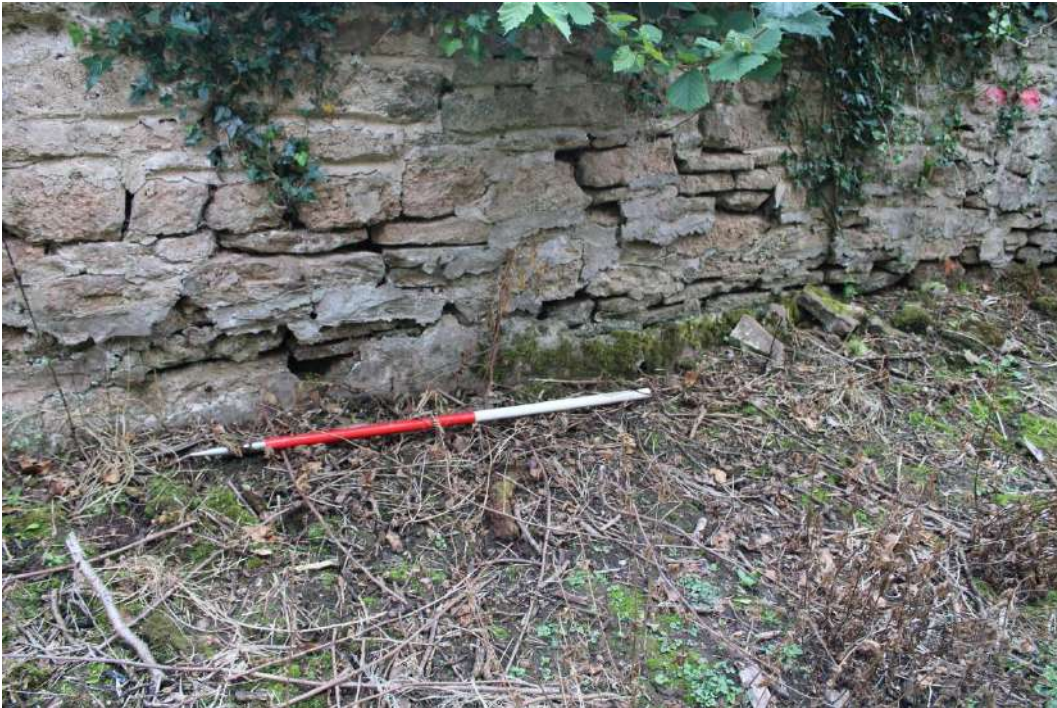
Photo 5: Detail of lower part of mill pond wall with possible metal sheet lining visible behind scale bar
