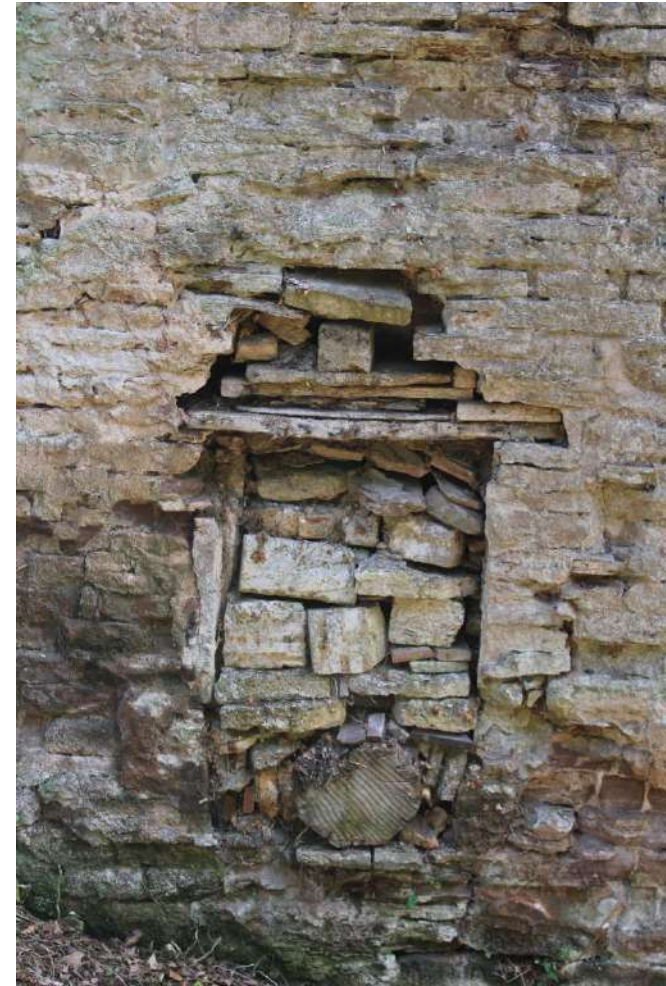
Photo 10: Detail of mill wheel housing and cut off axle visible at base
