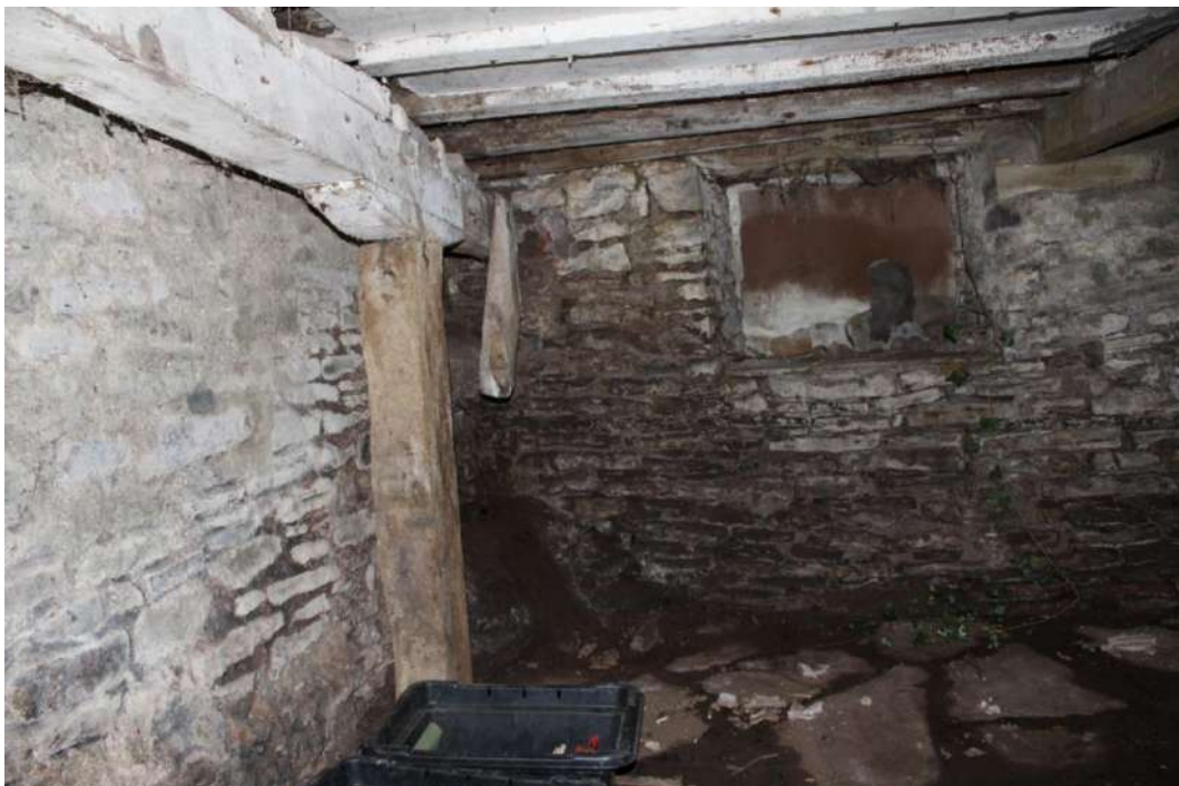
Photo 30: View into basement showing stone flagged floor and some areas of exposed bedrock through which the cellar has been excavated
