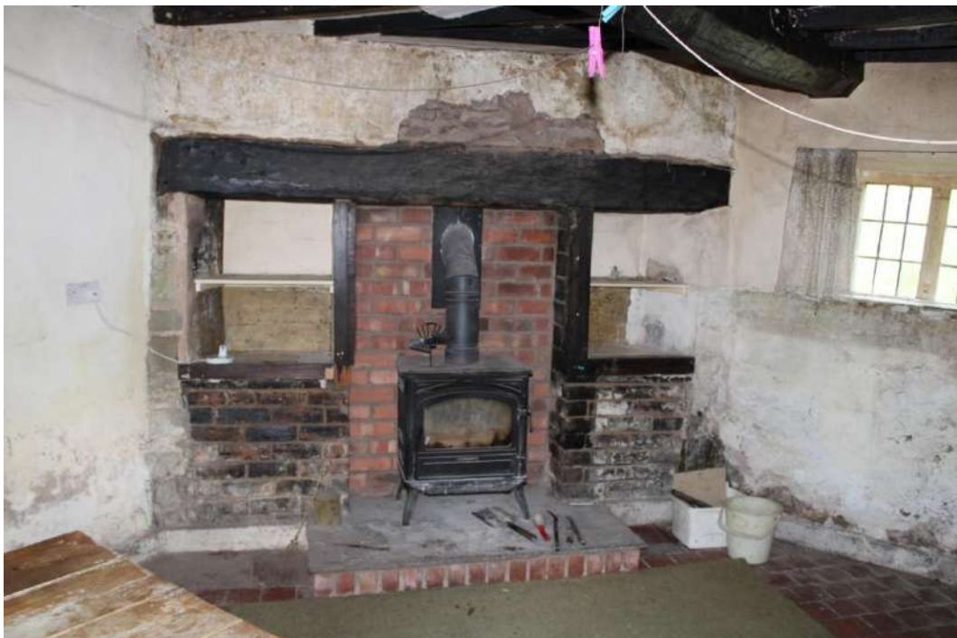
Photo 17: View of large fireplace in northeastern corner of northern ground floor room
