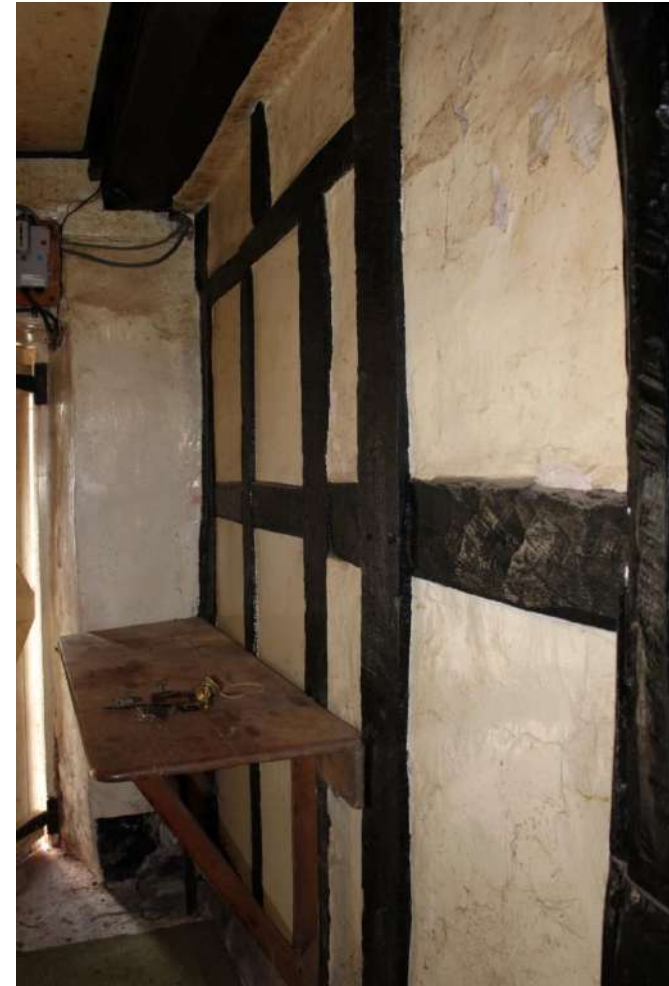
Photo 21: View of northern partition wall of central passageway looking southwest towards front door
